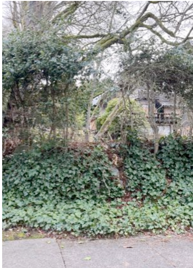
COLLAPSE IN EXISTING STONE WALL
