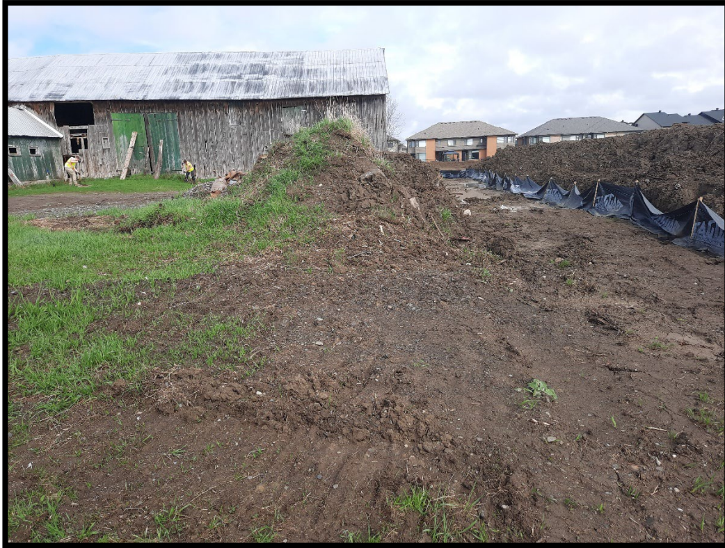
Figure 5: Example of disturbed conditions (MH1366-D013).
