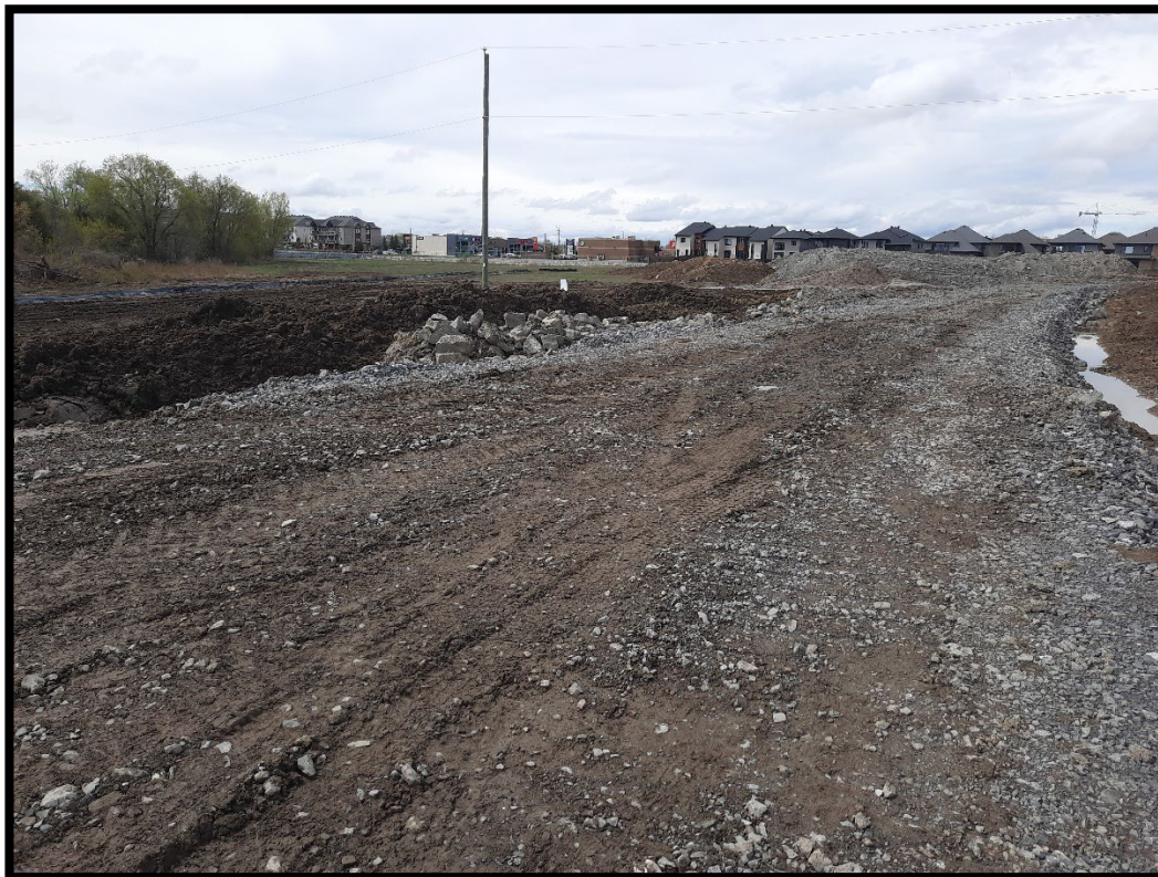
Figure 6: Example of disturbed conditions (MH1366-D050).
