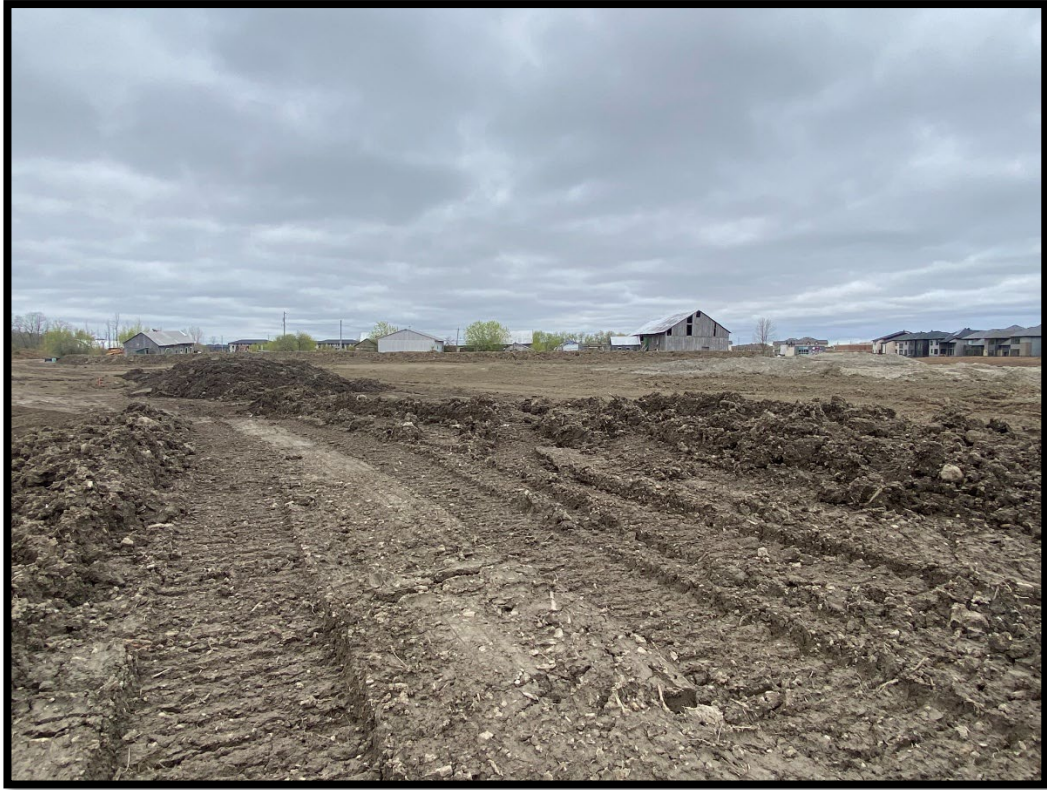
Figure 9: Example of disturbed conditions (MH1366-D083).
