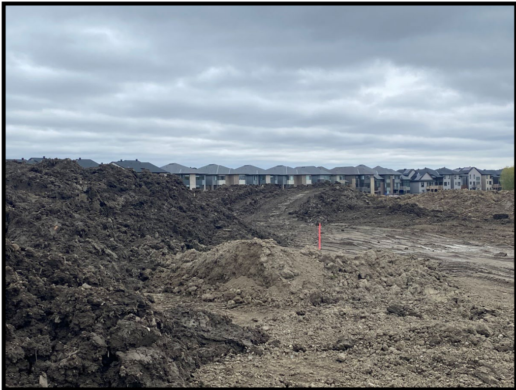
Figure 8: Example of disturbed conditions (MH1366-D081).
