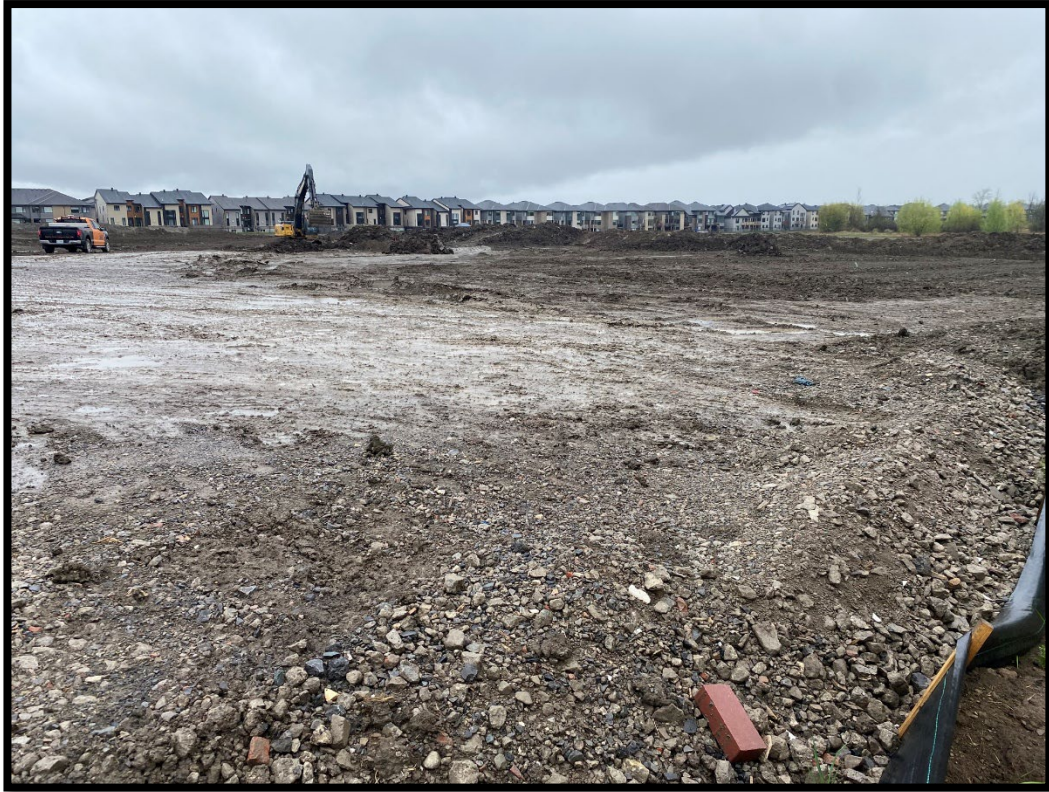
Figure 7: Example of disturbed conditions (MH1366-D068).
