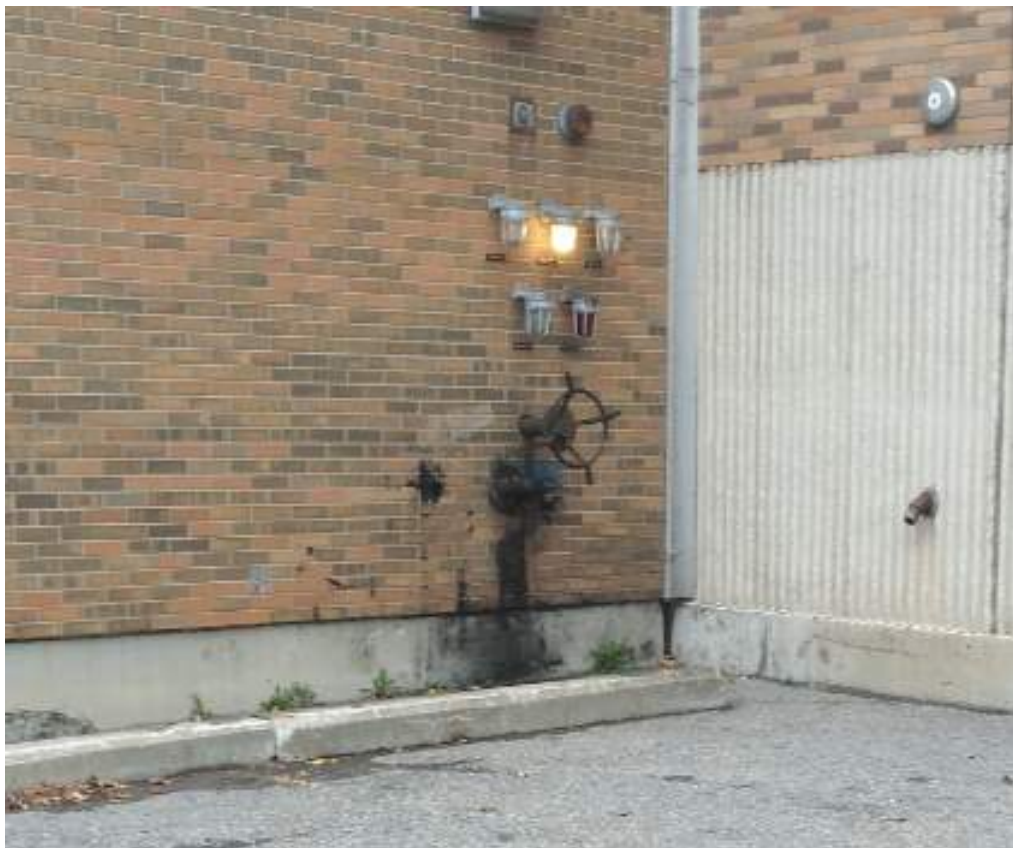
Photo 19: Stained brick and pavement with black ink at black ink fill pipes
