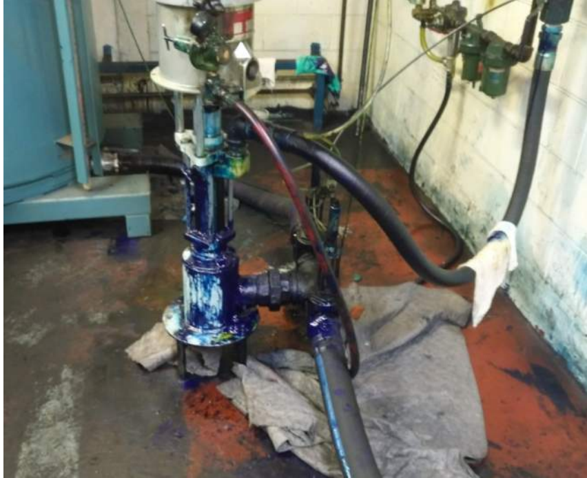
Photo 14: Coloured ink piping for dispensing
