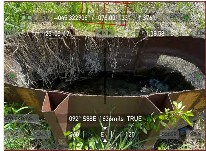
Site Photograph 6: The vertical drain on-site.
