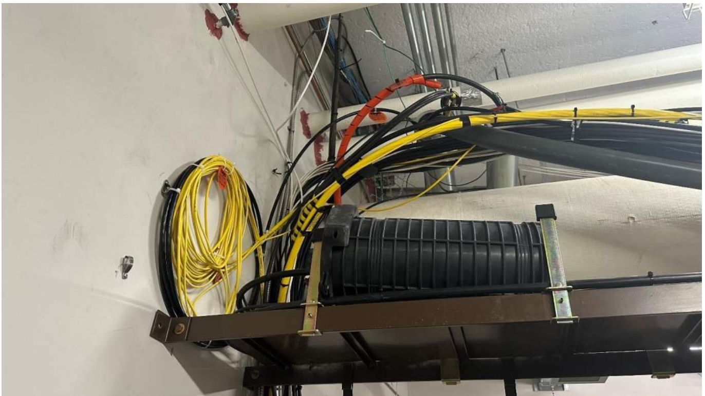
Image H.13: Brooke Claxton Building – IT Room Cabling Condition (1)
