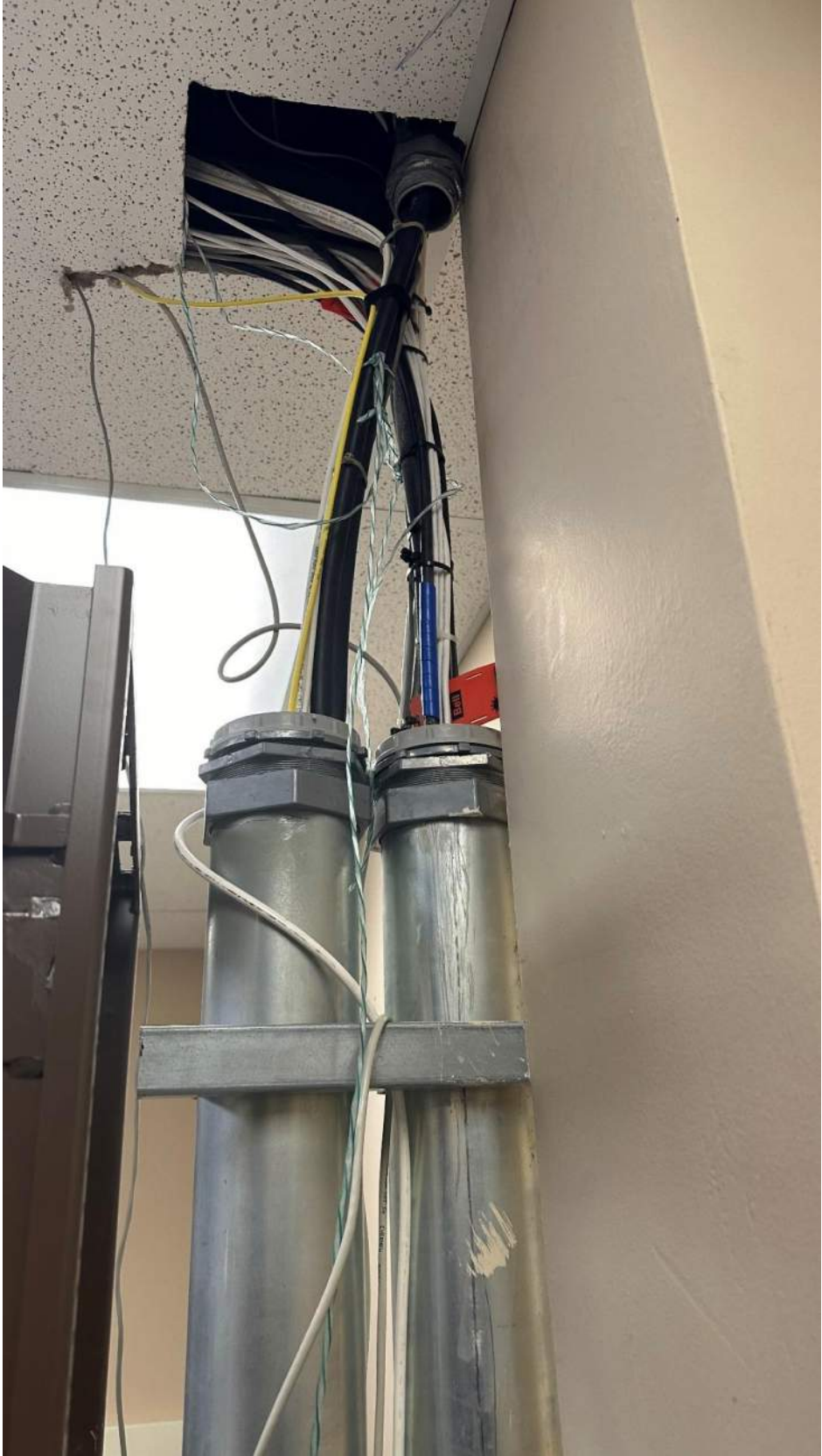
Image H.24: Standards Building – Cabling Entry Into IT Room
