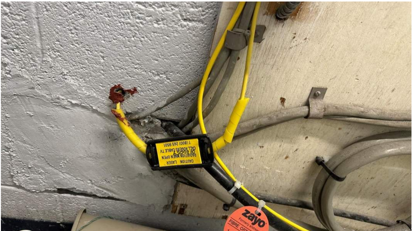
Image H.10: Personnel Records Building – Zayo Presence
