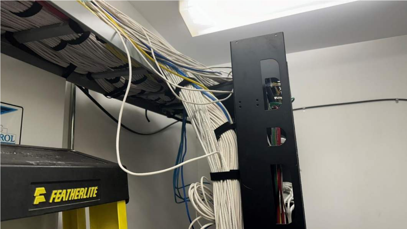
Image H.20: Occupational Health Unit – Pathways Incoming Into IT Room Rack
