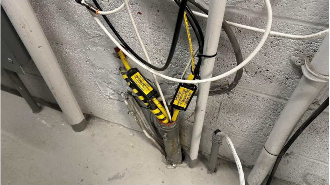
Image H.7: Personnel Records Building – Congested Pathways
