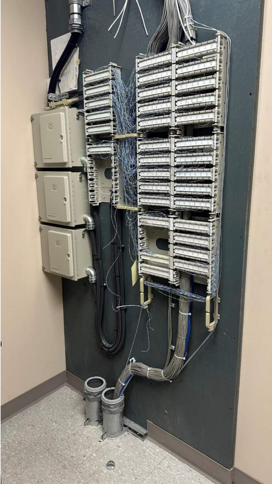
Image H.25: Standards Building – BIX Presence
