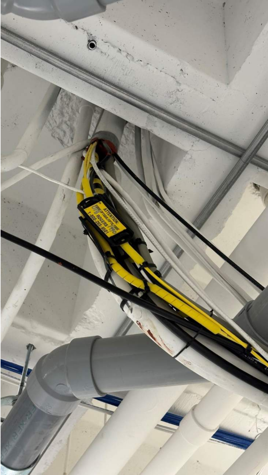
Image H.11: Personnel Records Building – Congested Pathways
