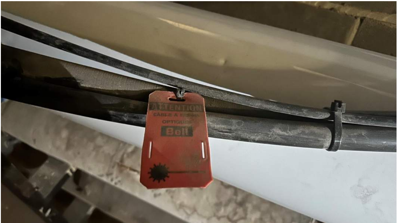
Image H.23: Standards Building – Bell Fibre Presence & Entry via Tunnel System
