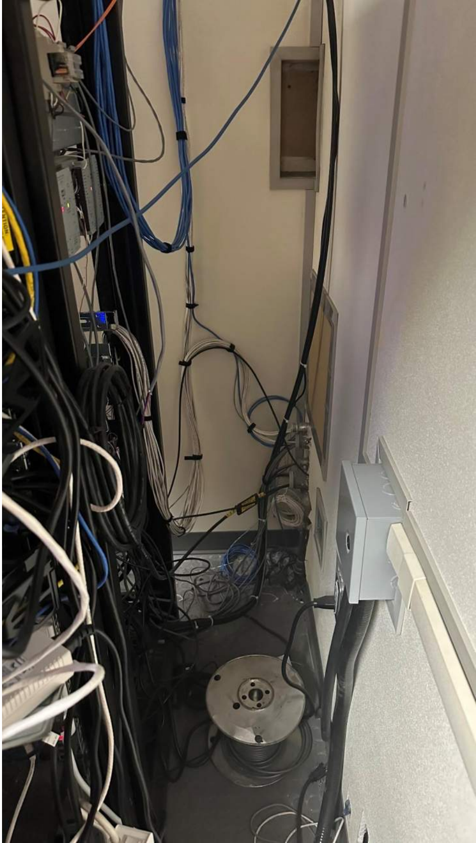
Image H.5: Heating & Cooling Plant – IT Room Condition
