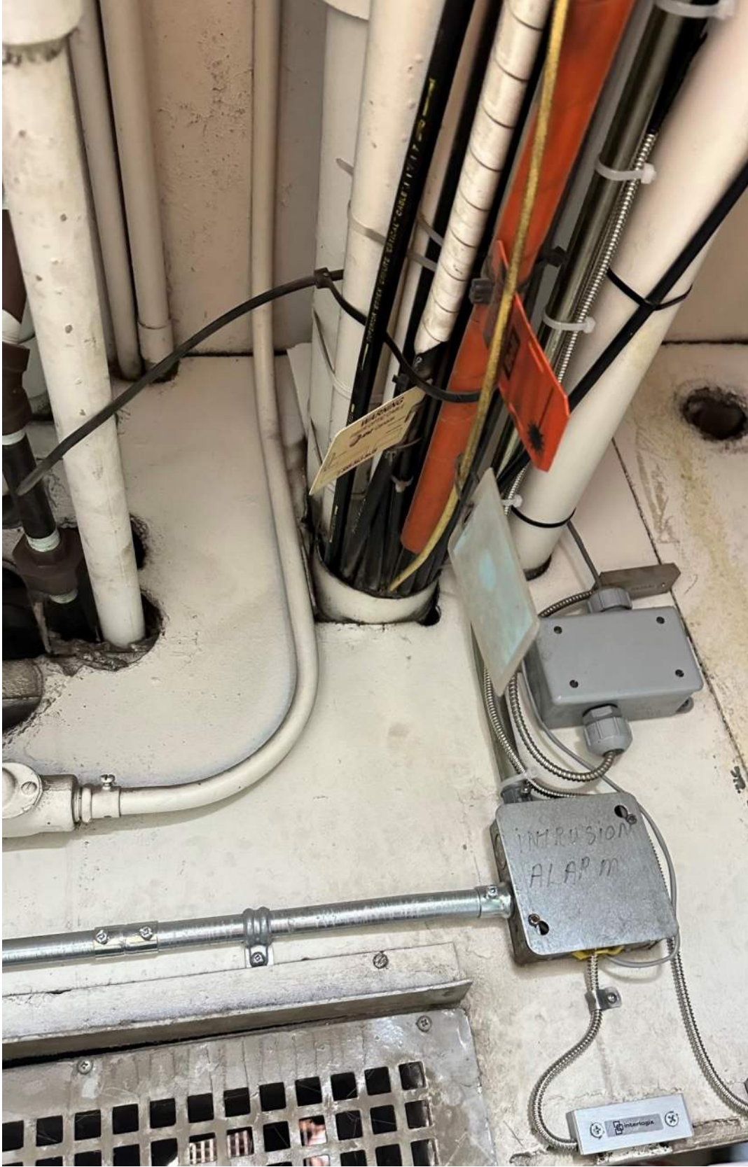
Image H.2: Heating & Cooling Plant - Congested Cabling (Ground Floor)
