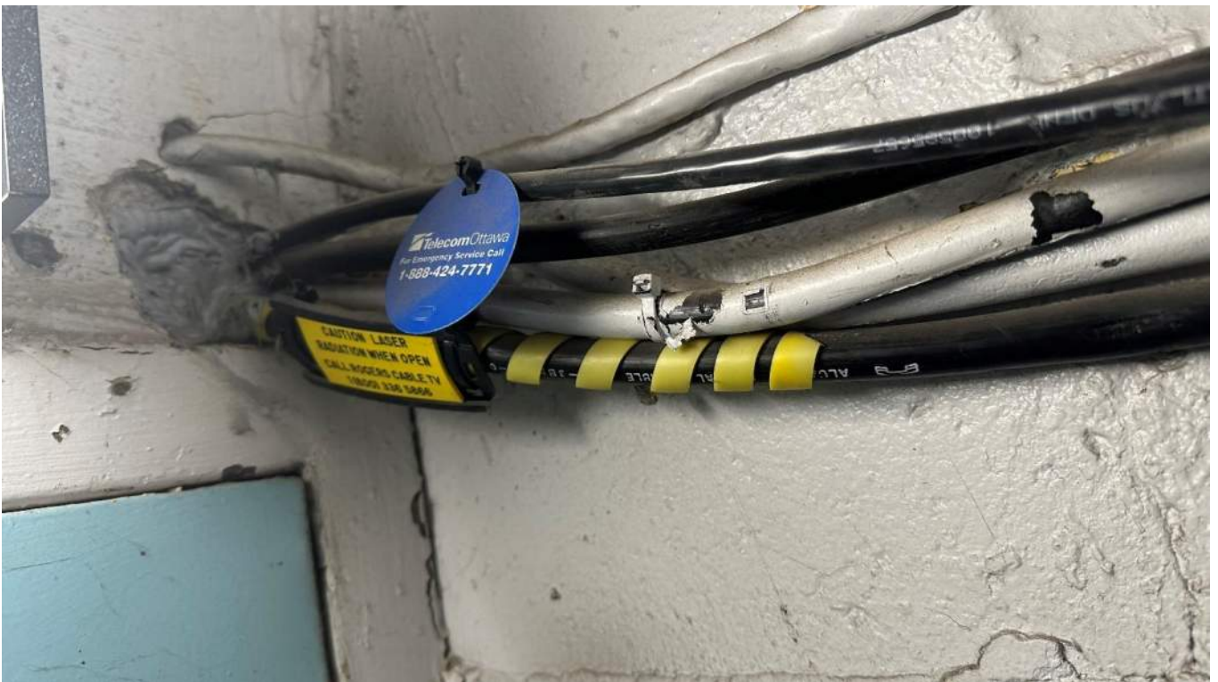
Image H.8: Personnel Records Building – Congested Pathways & Aging Cabling
