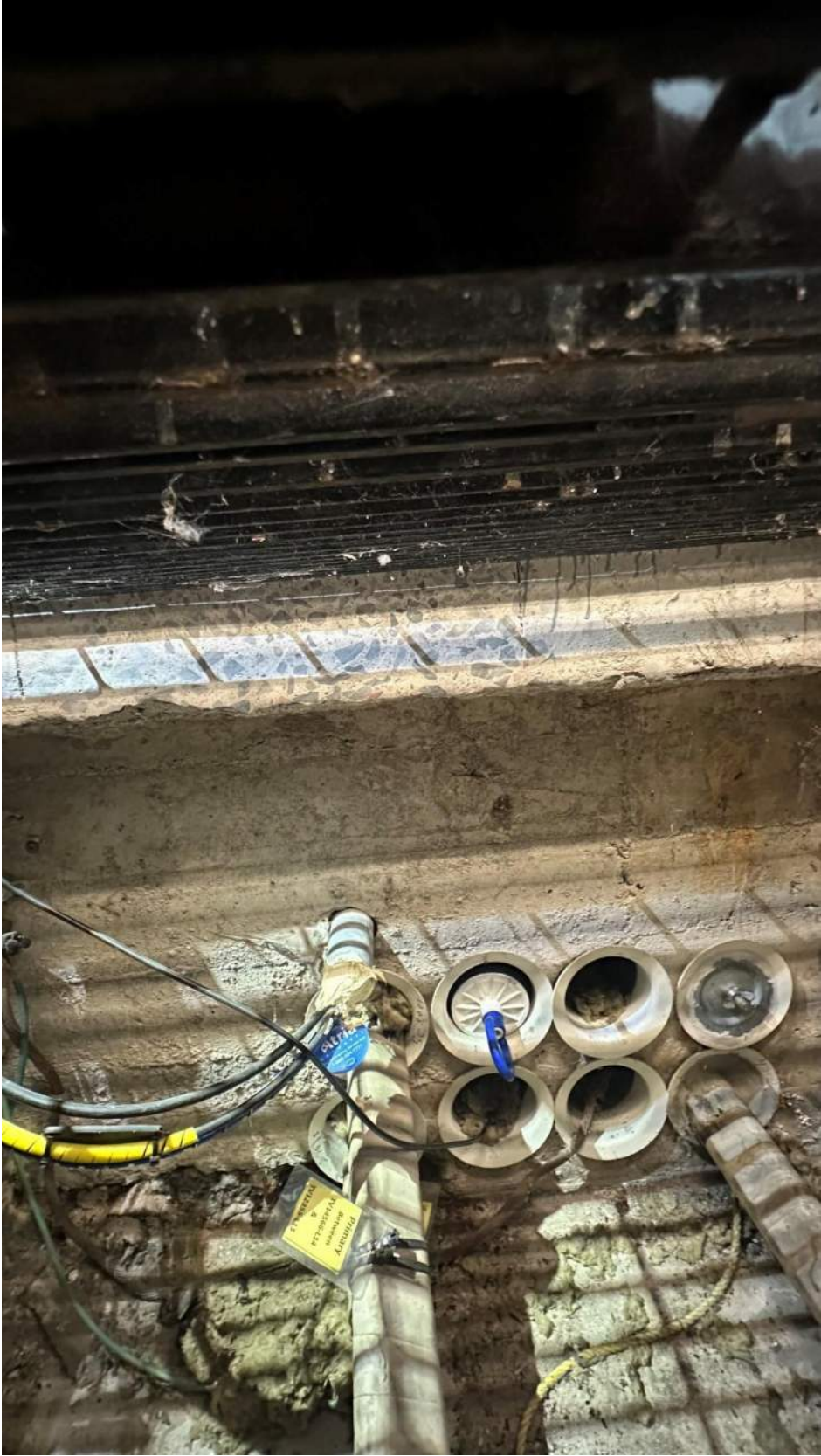
Image H.3: Heating & Cooling Plant – Duct Entry, West Side Interior
