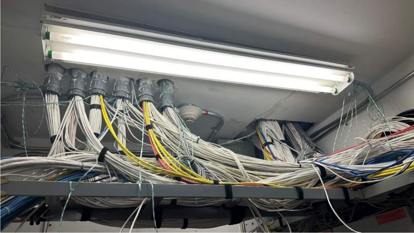
Image H.19: Occupational Health Unit – Pathways Incoming Into IT Room
