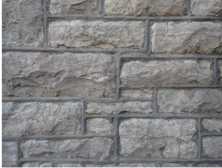
Figure 2: Detail capturing the condition of the limestone and mortar on the Stone Residence (Source: RMA+SH architects, 2026).
