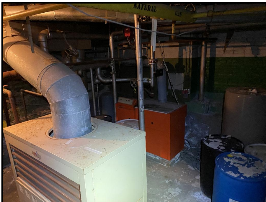
Photo 10: Mechanical room in the basement of the subject building.
