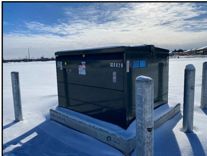
Photograph 6: Pad-mounted Hydro Ottawa transformer at northwest corner of Phase I Property.
