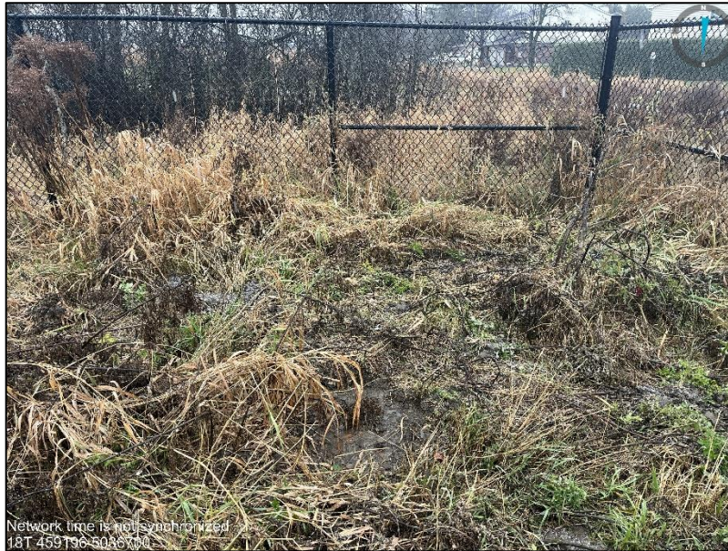
Municipal storm sewer manhole observed in the southwest portion of the Site
