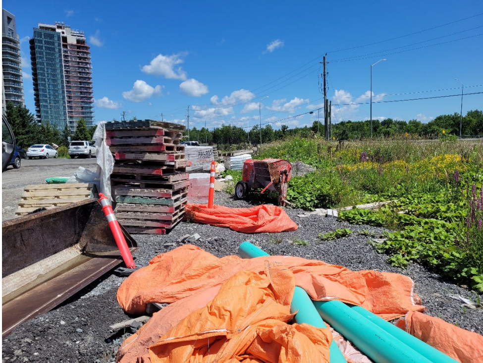
Photograph 5: View of the of the south portion of the Phase One Property looking east. View shows typical material storage for the adjacent construction project.
