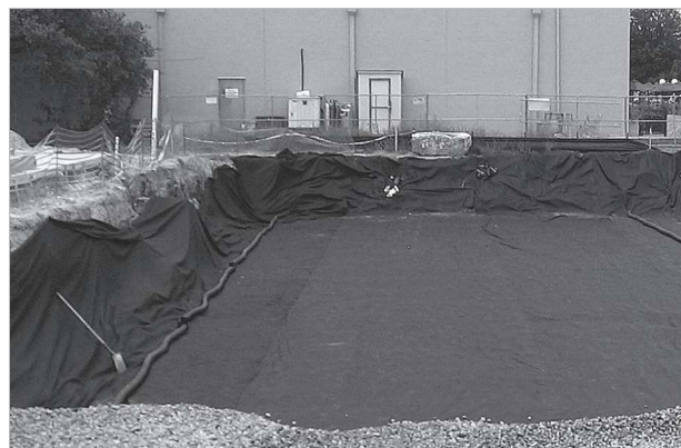
Place non-woven geotextile over prepared soils and up excavation walls. Install underdrains if required.
