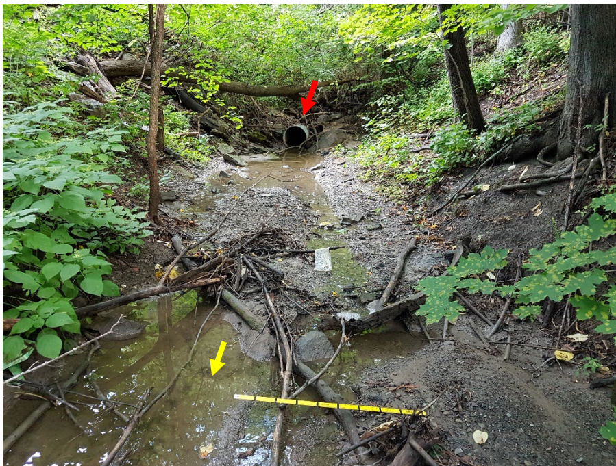
Flows conveyed through a compromised corrugated steel pipe that appeared overtopped during larger flows; however, erosion was not an issue.
