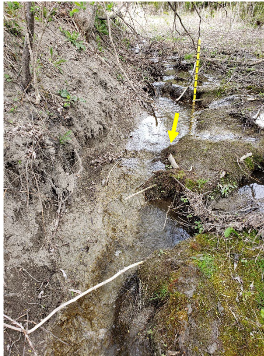
Example of exposed parent material at the toe of the valley slope, which is indicative of sloughing.
