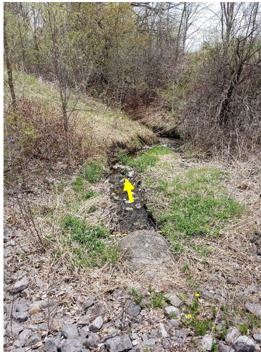
View of the channel downstream of the concrete culvert, where relatively minor channel adjustment along the toe of slope was observed.
