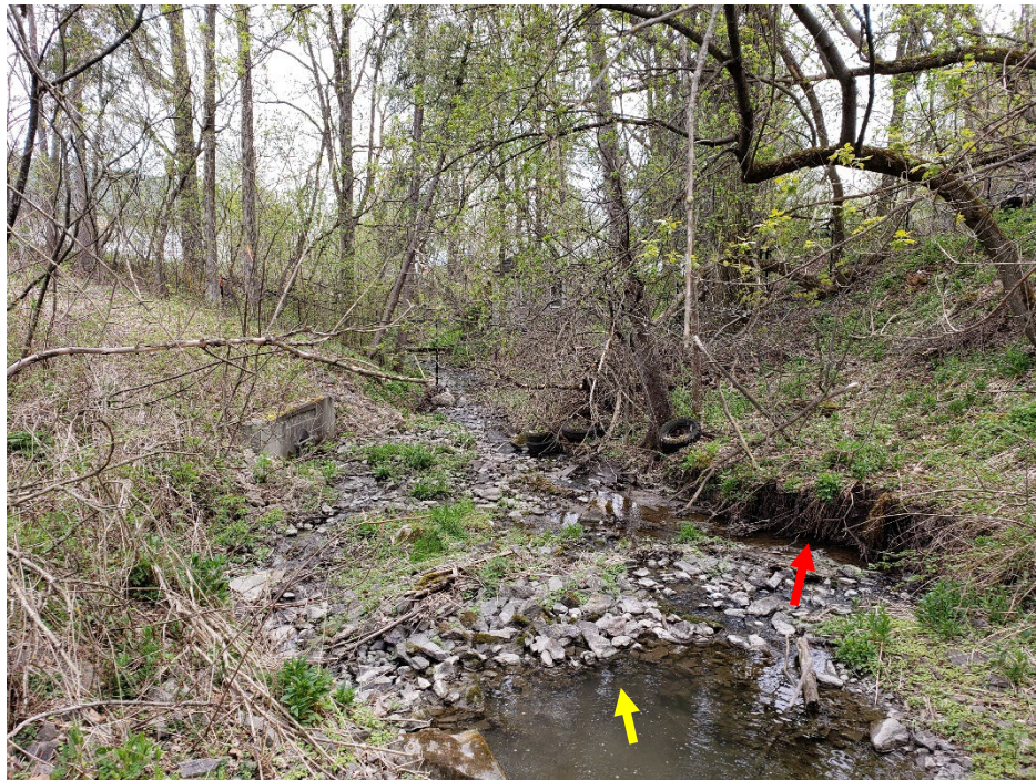
View of the channel downstream of the second concrete culvert. Relatively minor channel adjustment was observed along the toe of slope (red arrow).
