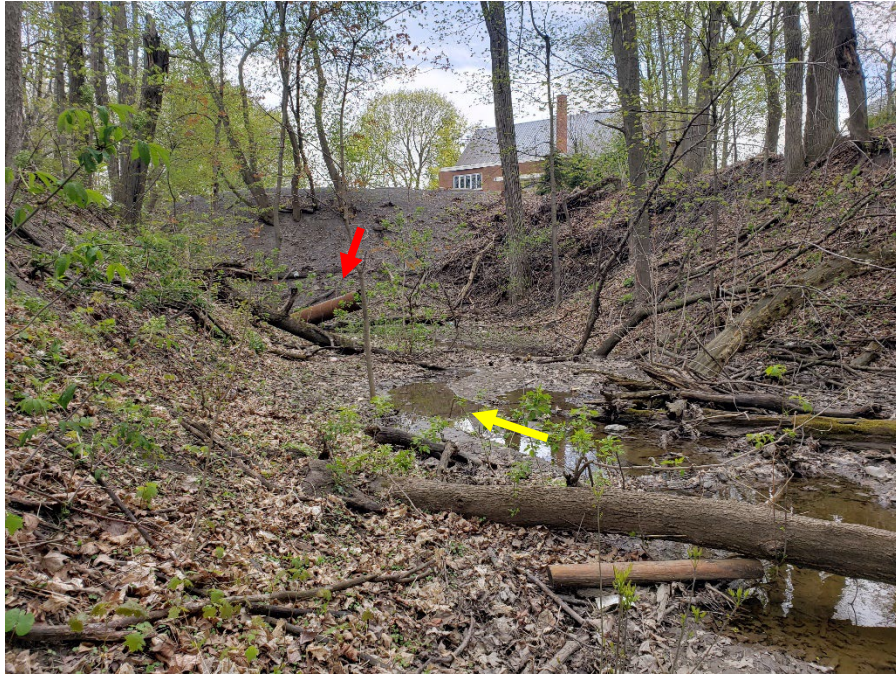
View of the ravine adjacent to the church where the channel was poorly defined and the majority of trees on the slope were upright. The location of the damaged CSP culvert is shown by the red arrow.
