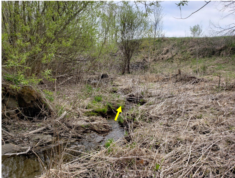
View of the channel approaching the first concrete culvert installed as part of an online stormwater management facility.
