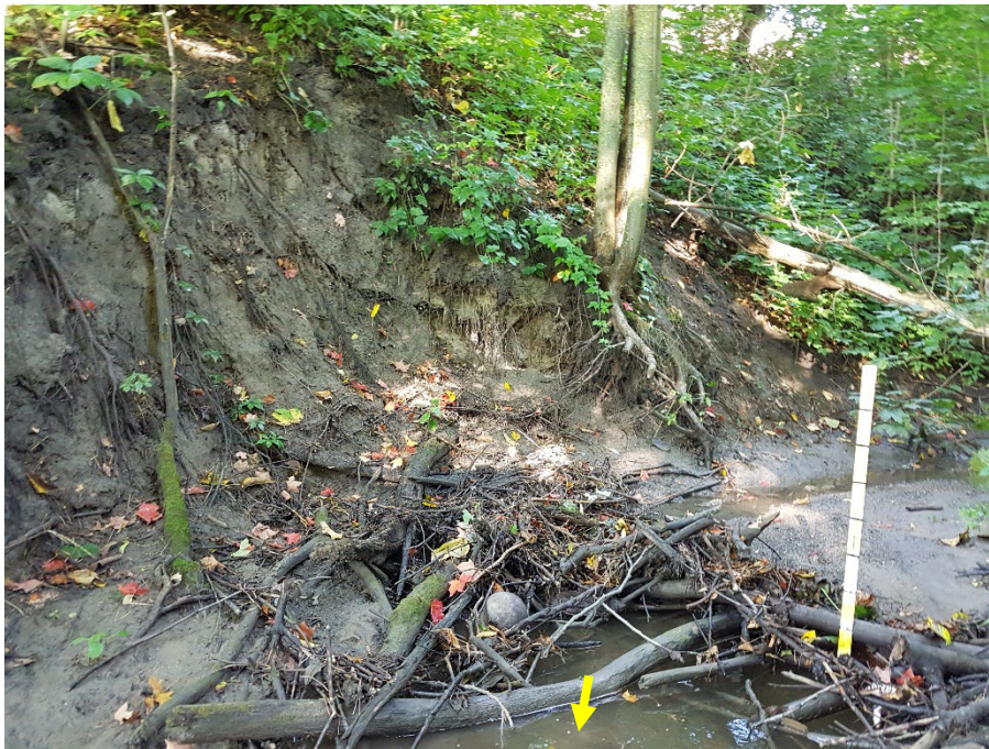
Eroded bank opposite the proposed development with a moderately dense root network. Several woody debris jams were present throughout the downstream extent of the reach.
