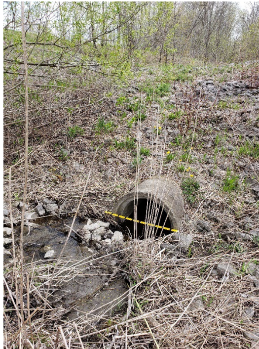
View of the culvert inlet. The control structure was stable, with no evidence of outflanking or overtopping.
