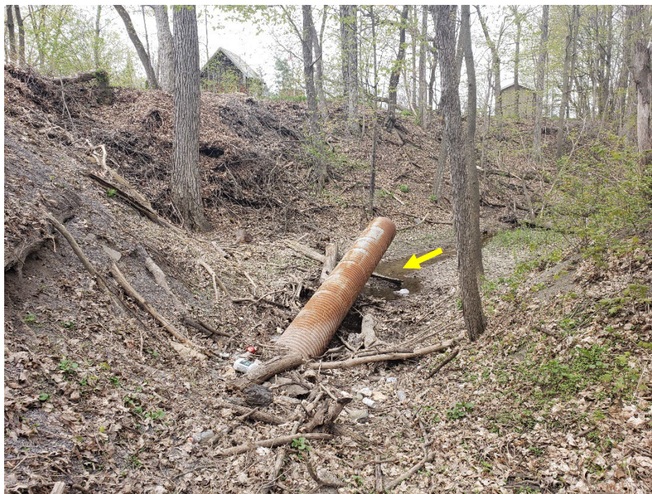
View of damaged CSP with the inlet suspended approximately 0.9 m above the channel. Flows appear to enter the culvert through hole(s) approximately midway in the structure.
