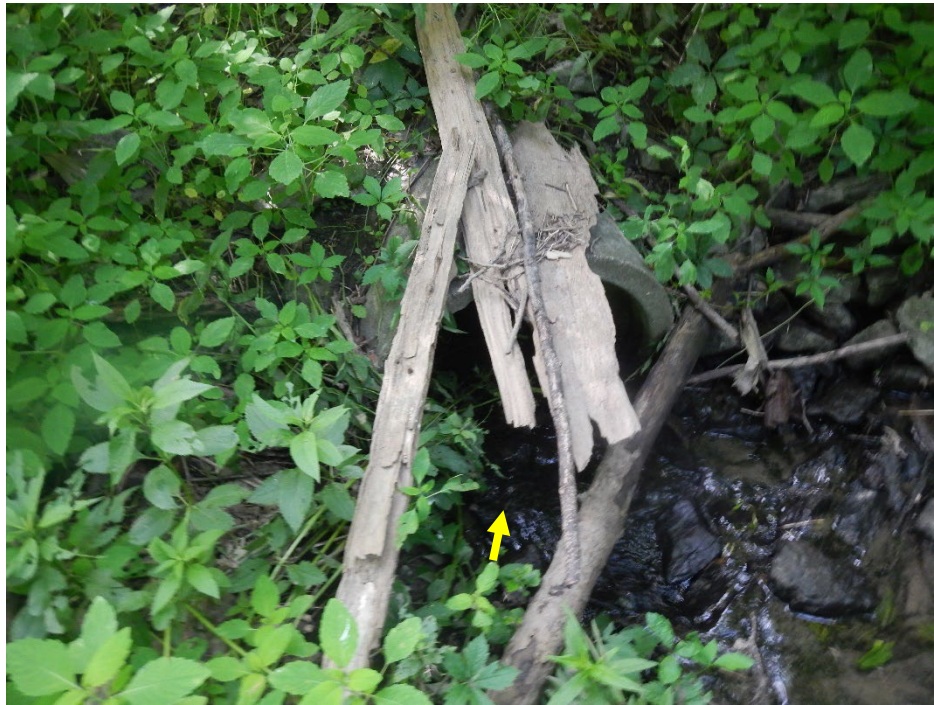
Concrete culvert located in the lower third of the reach. Rip rap stabilization was observed on top of the culvert. No channel adjustment was observed in vicinity of the crossing.
