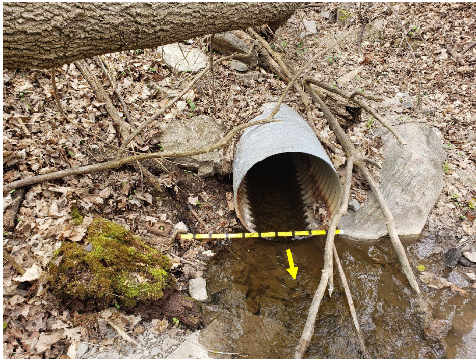
Downstream end of damaged corrugated steel pipe culvert (also pictured in Photo 36). Recent disturbance to the ravine was evident through the placement of fill near the top of slope to the west and debris on the slopes.
