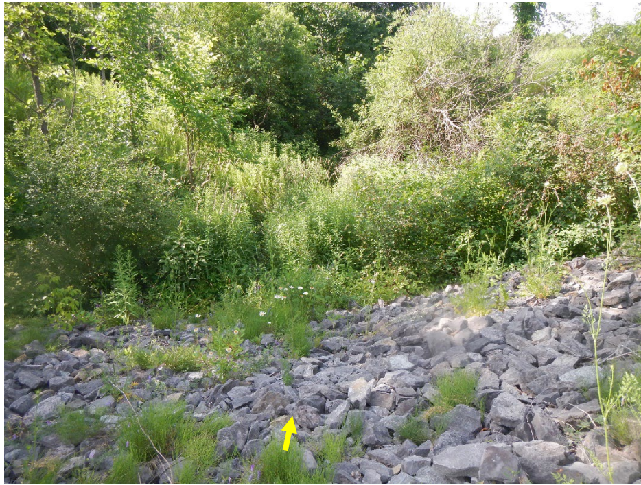
Riprap stabilization on top of a concrete culvert in the upper third of the reach. Note the channel remained extensively encroached with vegetation and flowed through a confined valley. No erosion was observed in vicinity of the crossing.
