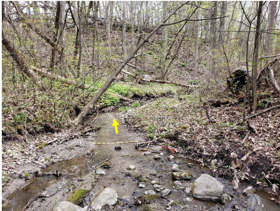
The majority of trees in the valley and on the slopes were upright, suggesting that the reach was relatively stable. The channel was positioned away from the valley toe.
