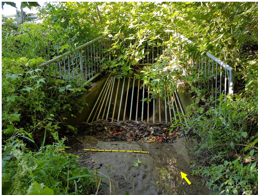
Downstream extent of the reach at Carp Road, where the tributary flowed into a 0.90 m diameter concrete pipe.
