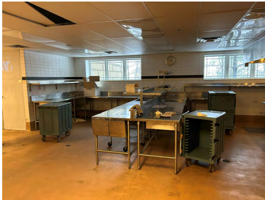
Photo 8 View of the kitchen located on the first level of the Site building.
