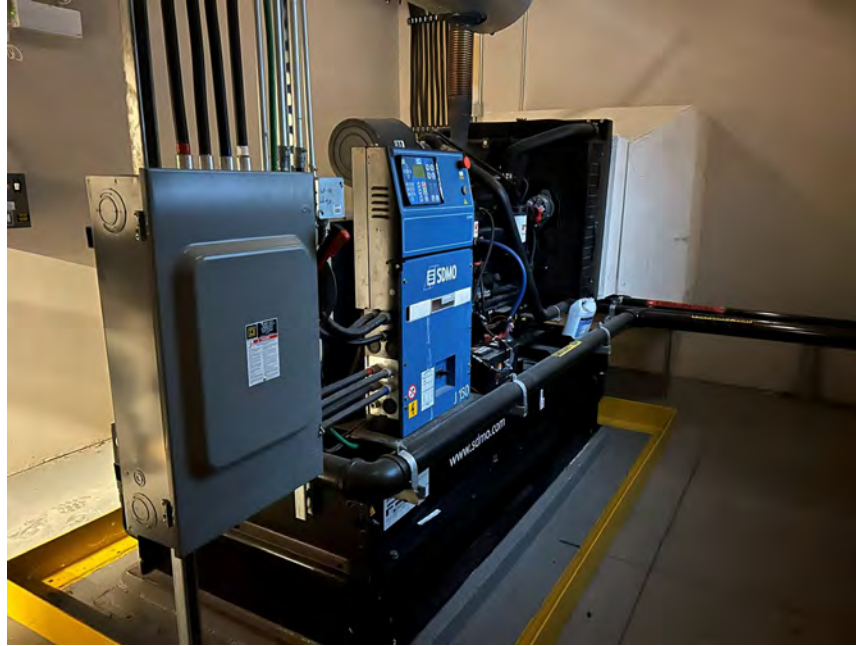
Photo 15 View of diesel-powered back-up generator with integrated 450-litre diesel AST in the generator room in the western portion of the Site building.
