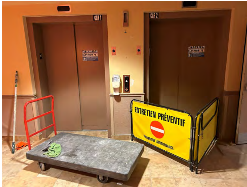
Photo 3 Photo showing two of the three hydraulic elevators in the Site building.
