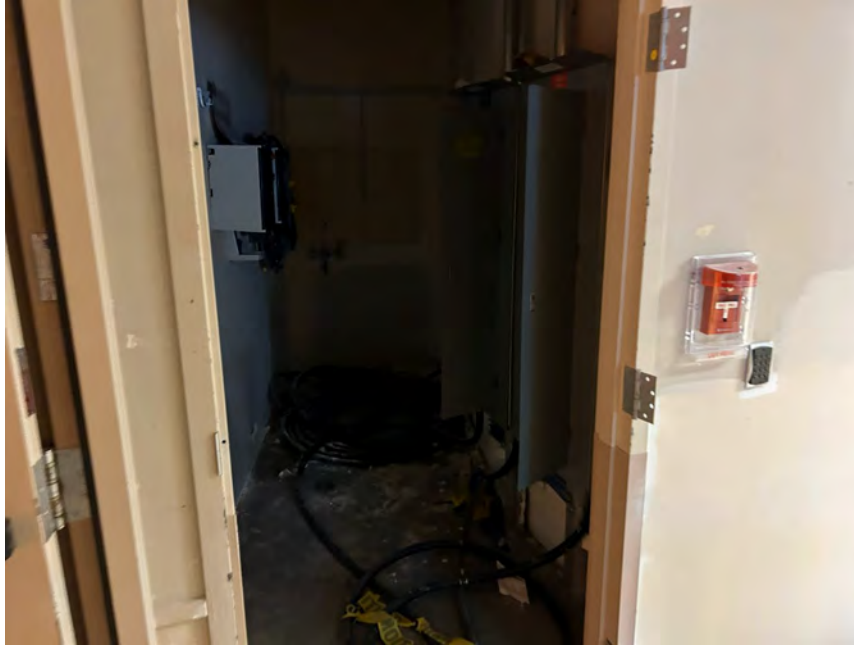
Photo 11 View of the elevator mechanical room and sump on the first level of the Site building, lighting was non-operational.
