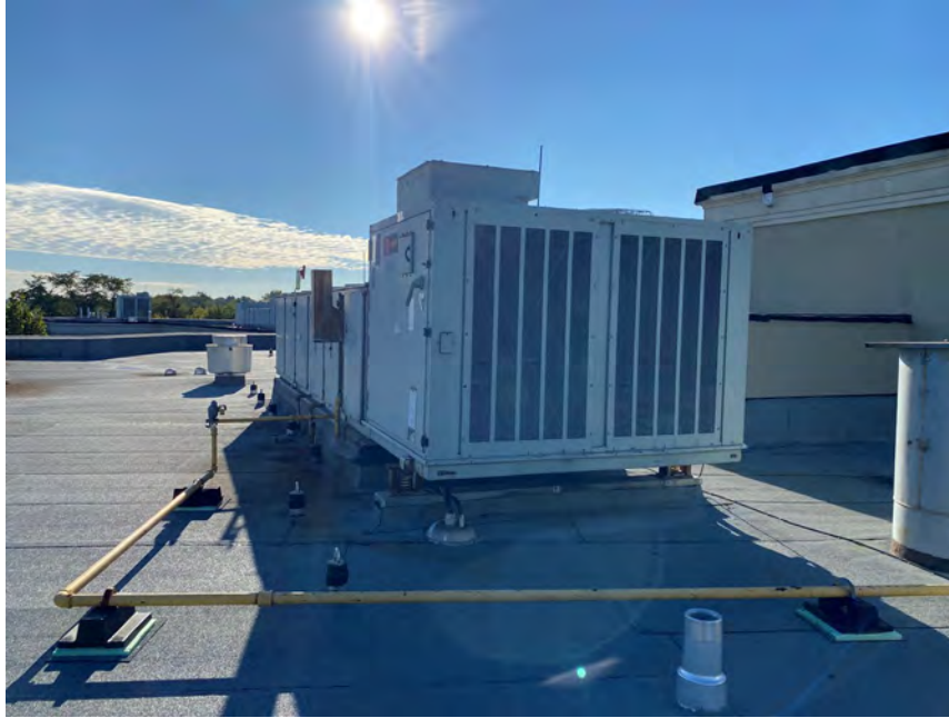
Photo 13 View of a natural gas-fired roof-mounted HVAC unit in the Site building (2024).
