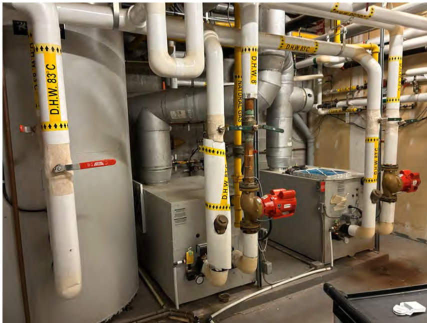
Photo 14 View of the natural gas-fired hot water heaters in the mechanical room on the first level of the Site building.
