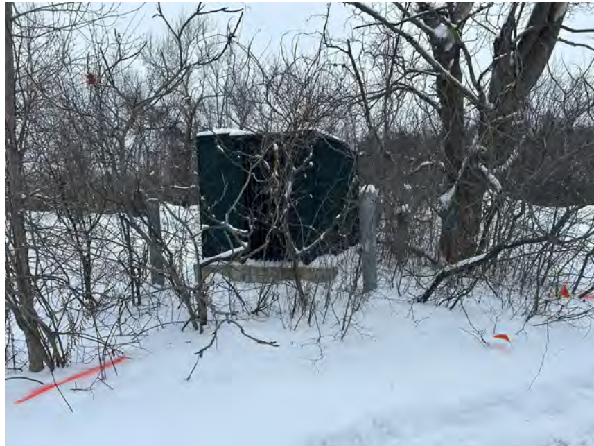
Photo 18 View of the pad-mounted transformer at 1533 Property parcel, facing northwest.
