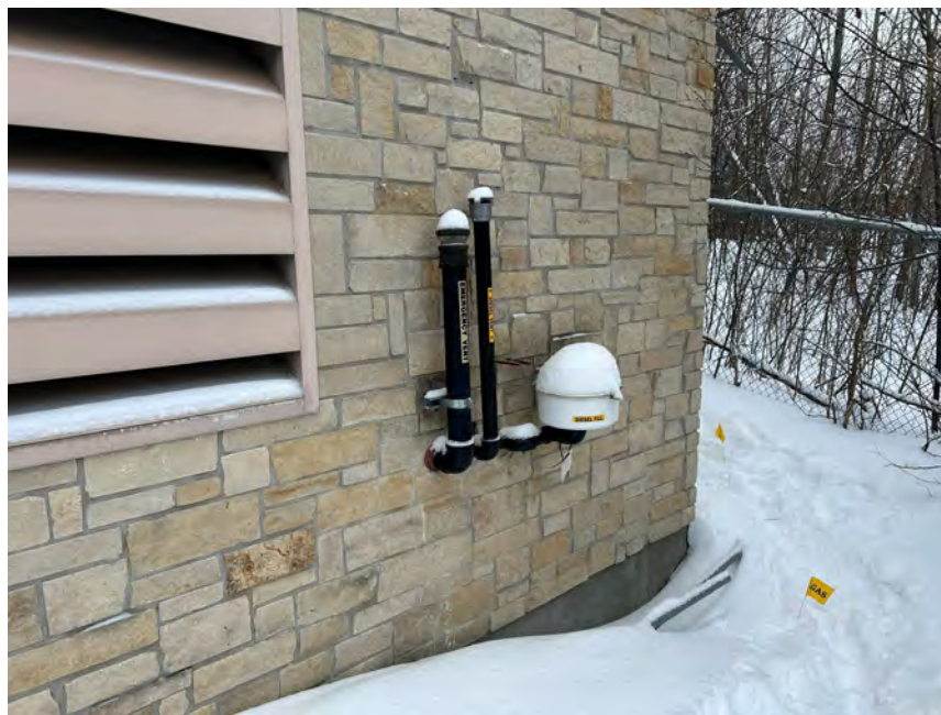
Photo 16 View of the exterior fill pipes for the diesel back-up generator AST, facing southeast.
