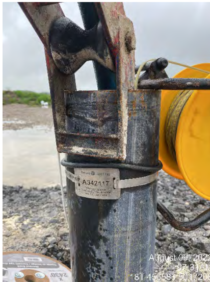
Photo 3 - Wellhead at pumped water well A342117.
