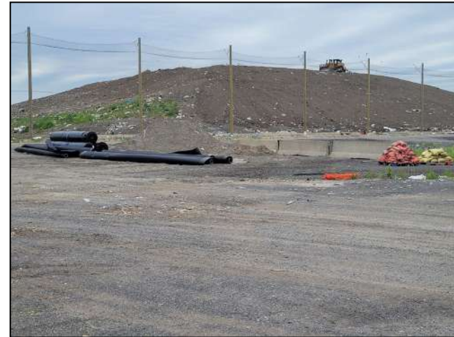
Photo 14: View of active fill area northwest of site (Photo taken looking northwest).
