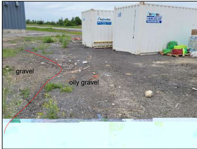
Photo 13: Example of oily gravel placed at the site (Photo taken looking southeast).
