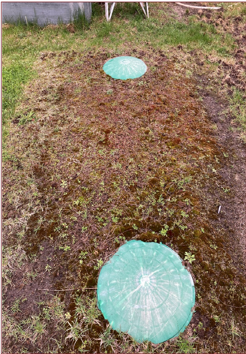
Photograph 31: Septic Tank for CACE Construction portable.
