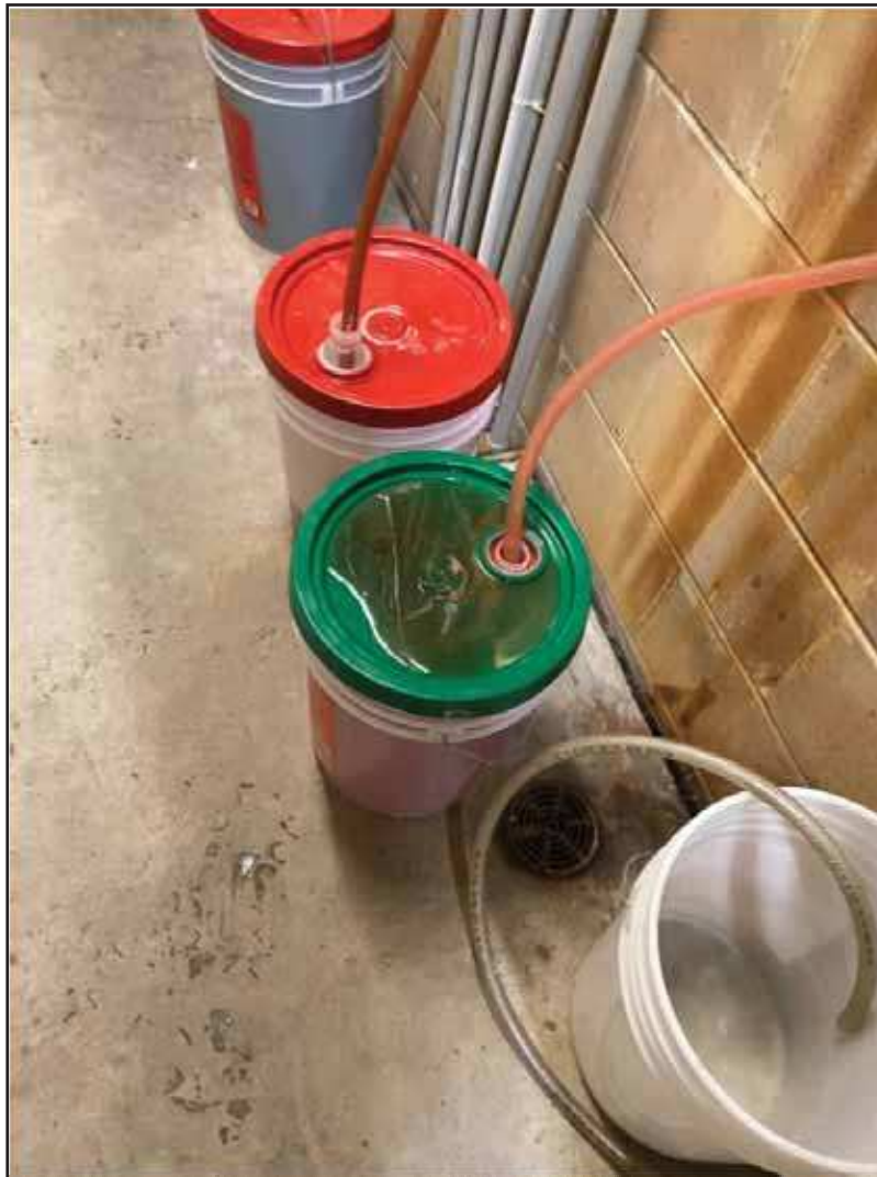
Photograph 11: View of concentrated cleaning liquids for the car wash. A floor drain is pictured.
