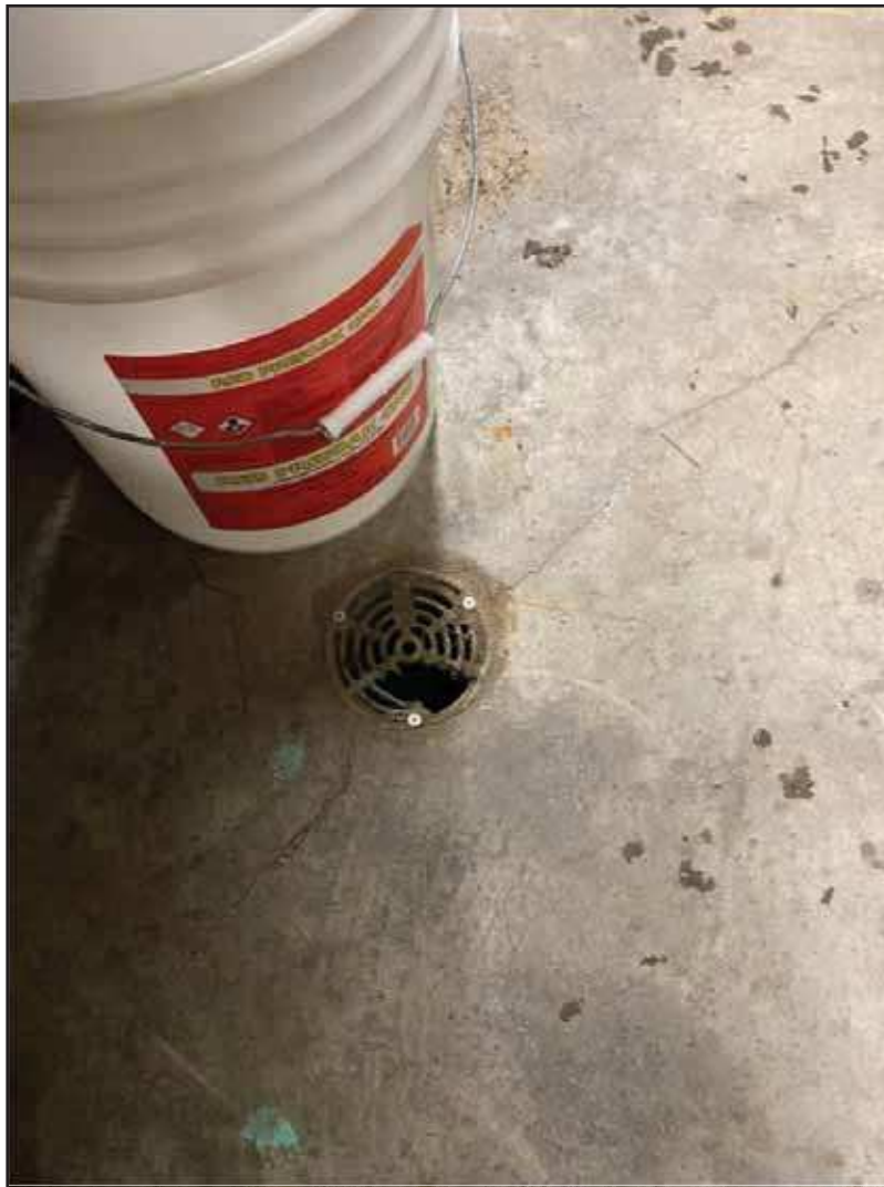
Photograph 16: View of floor drain near the entrance to the car wash.
