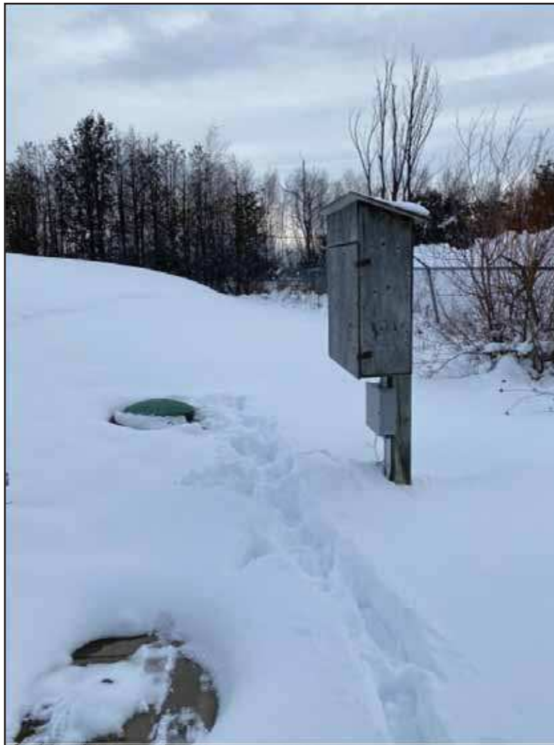
Photograph 5: View of access hatches and electrical systems associated with the septic system located on the south property boundary.
