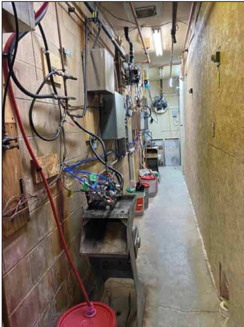
Photograph 10: Interior view of the car wash. Mechanical systems for the car wash are pictured.
