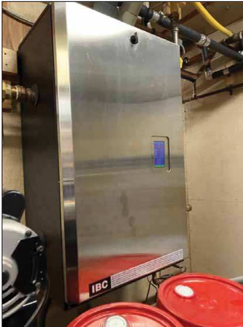
Photograph 13: View of car wash heating system.
