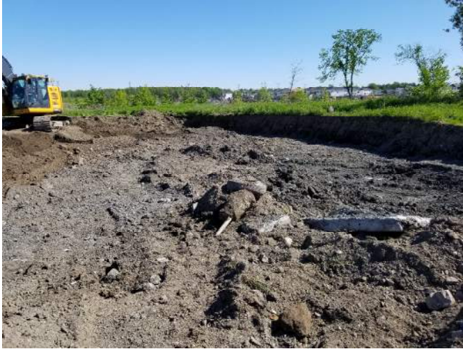
PHOTO 1: Remedial Excavations showing the removal of construction debris and soil piles for off site disposal.
