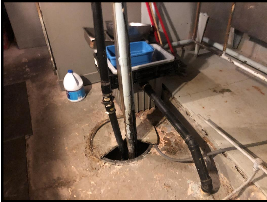
Photograph 7: Sump pump located in basement addition of 91 Holland Avenue, facing east.
