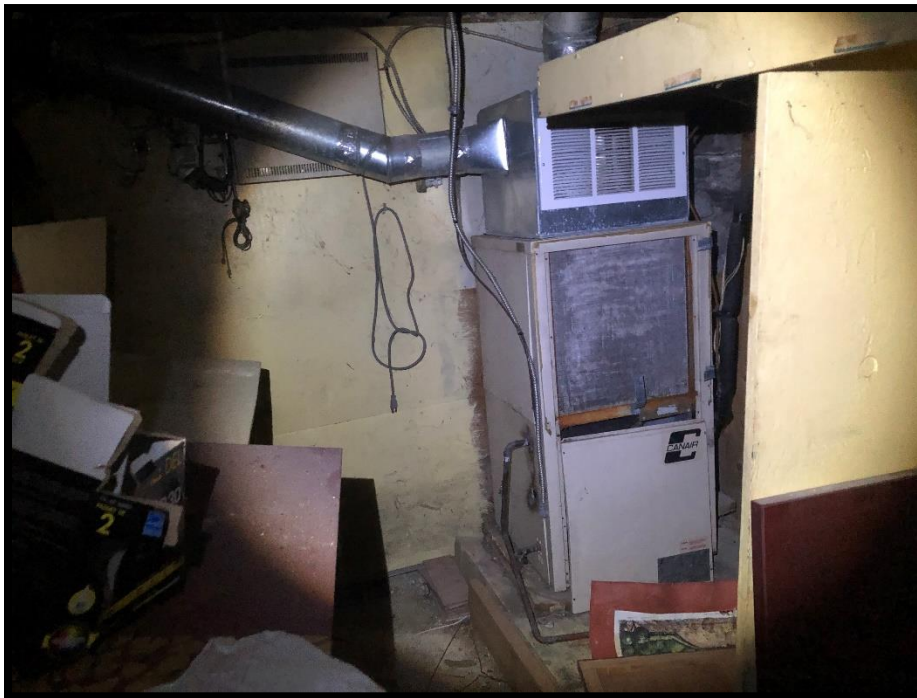
Photograph 8: Natural gas-fired furnace in basement of 91 Holland Avenue, facing west.
