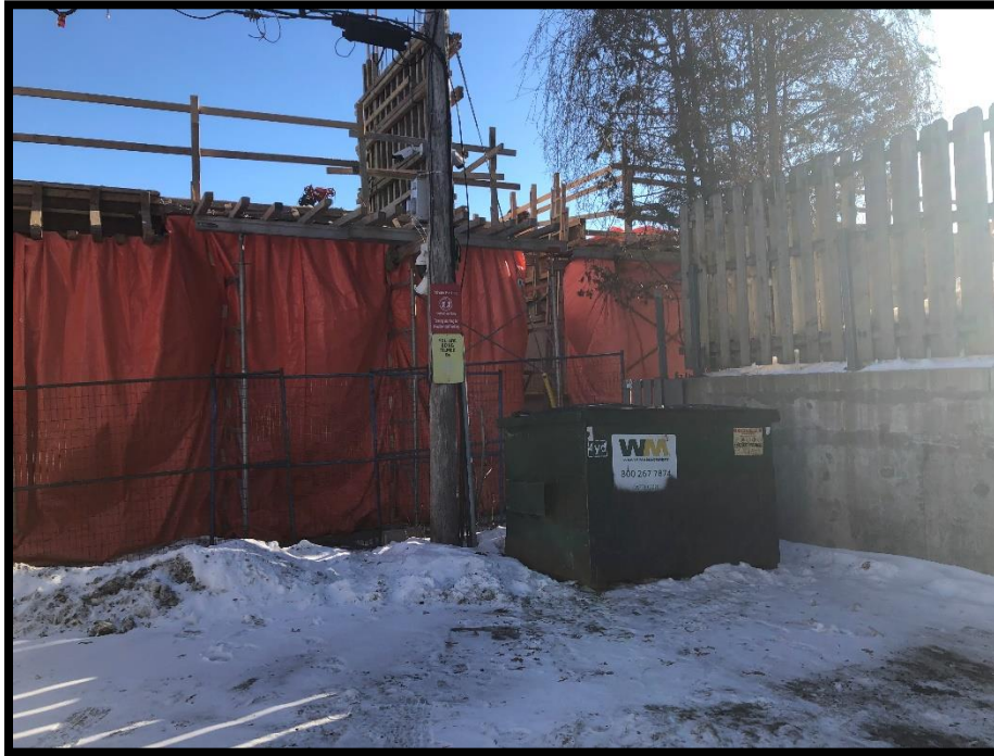
Photograph 3: Waste bin at rear parking area of 93 Holland Avenue showing ongoing construction to the east, facing southeast.
