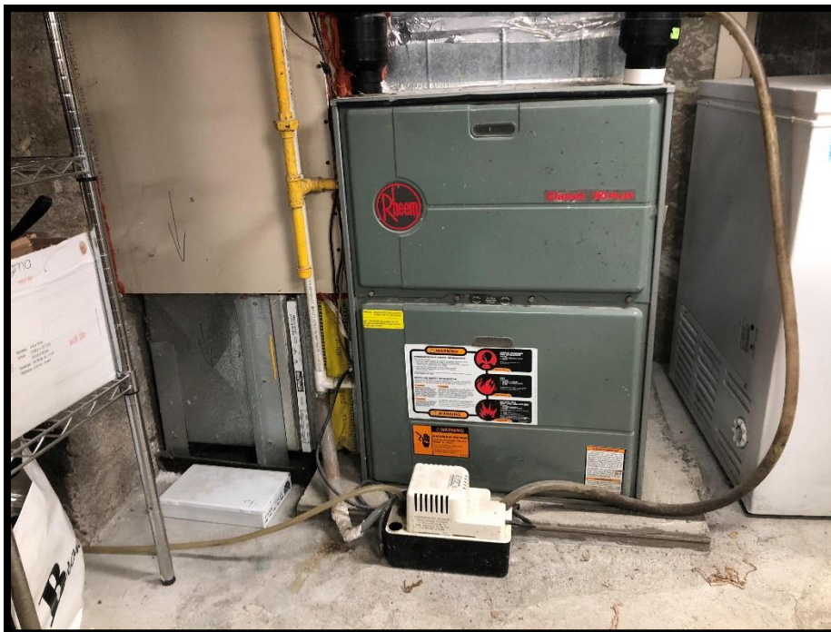
Photograph 4: Natural gas-fired furnace in basement of 93 Holland Avenue, facing south.
