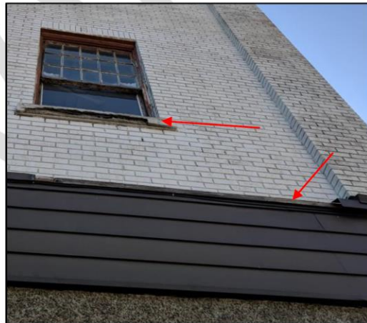
Photo 8: Deteriorated concrete window sill and damaged flashing on west elevation [JCAL 2018].
