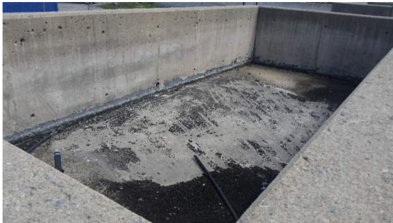
Photo 8 – Former planter on the second floor of the parking garage (facing southeast).
