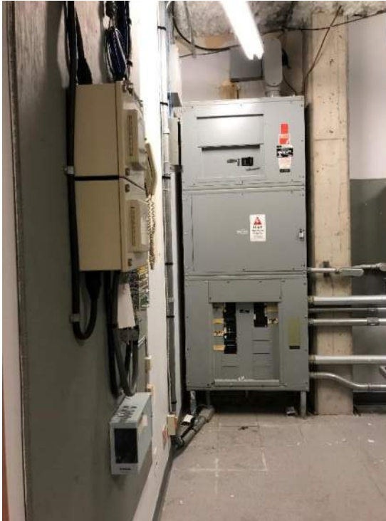
Photo 13 - View of the electrical room on the lower level of the building
