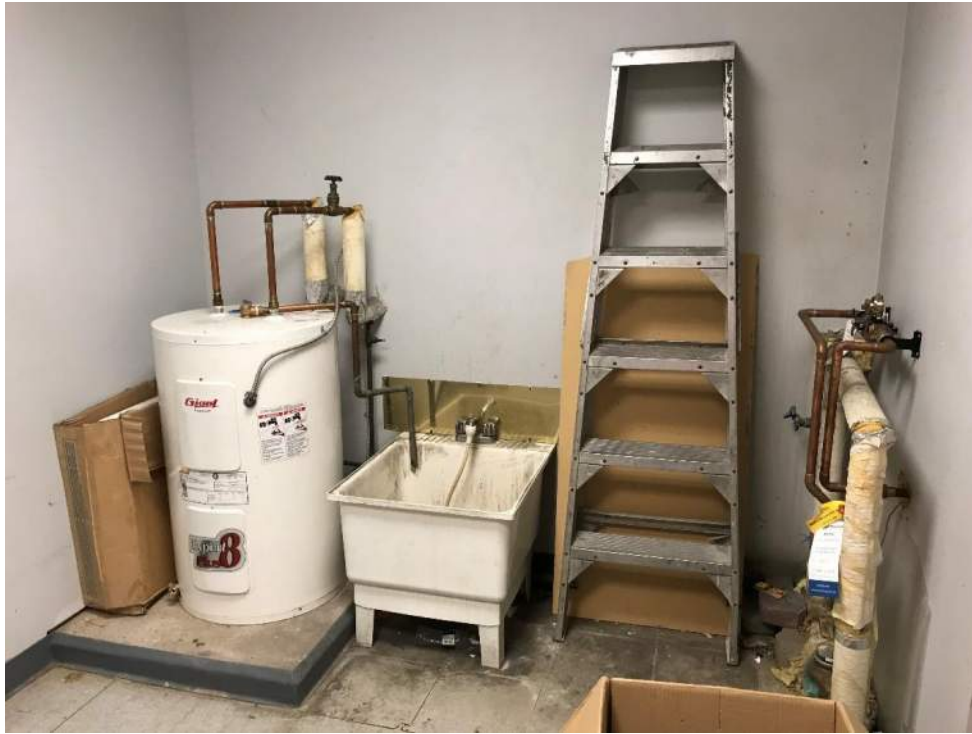
Photo 11 - View of the water supply pipes and the hot water tank
