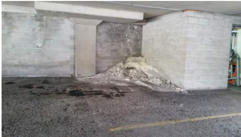
Photo 17 – Salt in the first floor of the parking garage (facing north).
