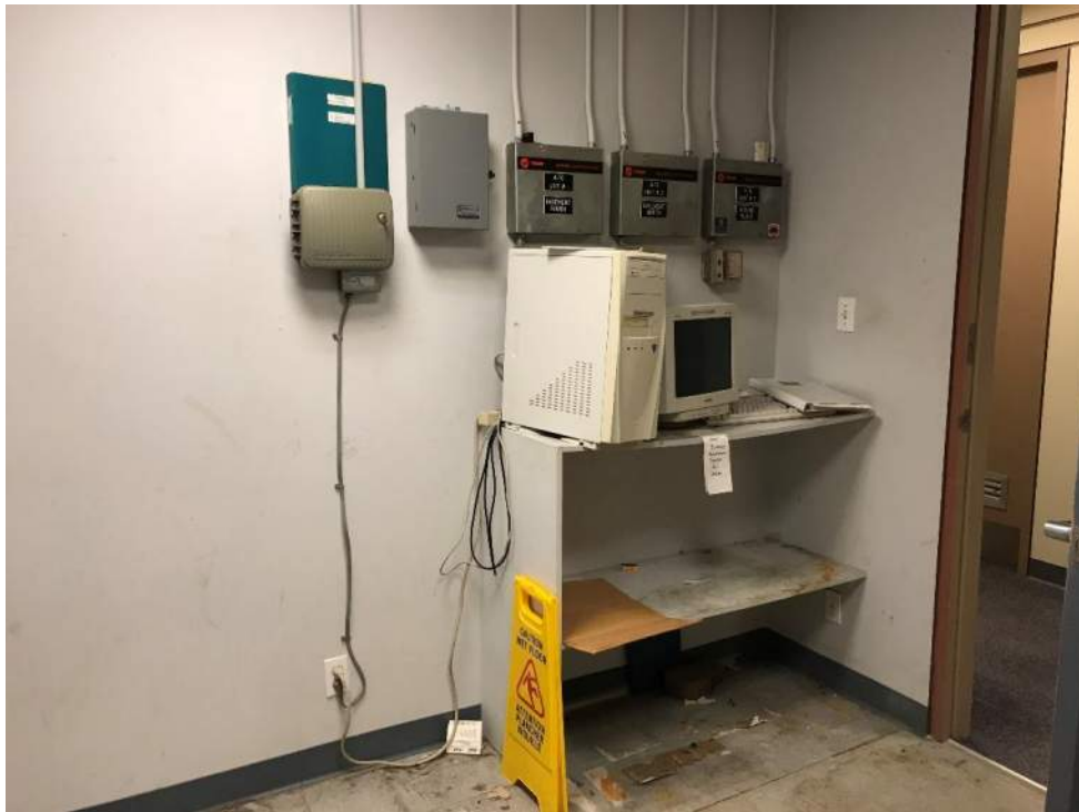
Photo 12 – View of the HVAC controls
