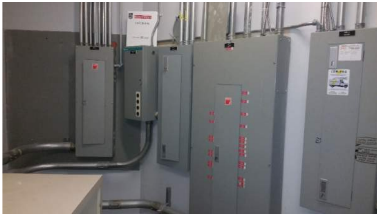
Photo 12 – Electrical room on the first floor of the RBC.
