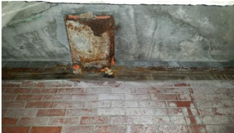
Photo 15 – Salt staining on the wall of an empty storage room on the first floor of the parking structure.
