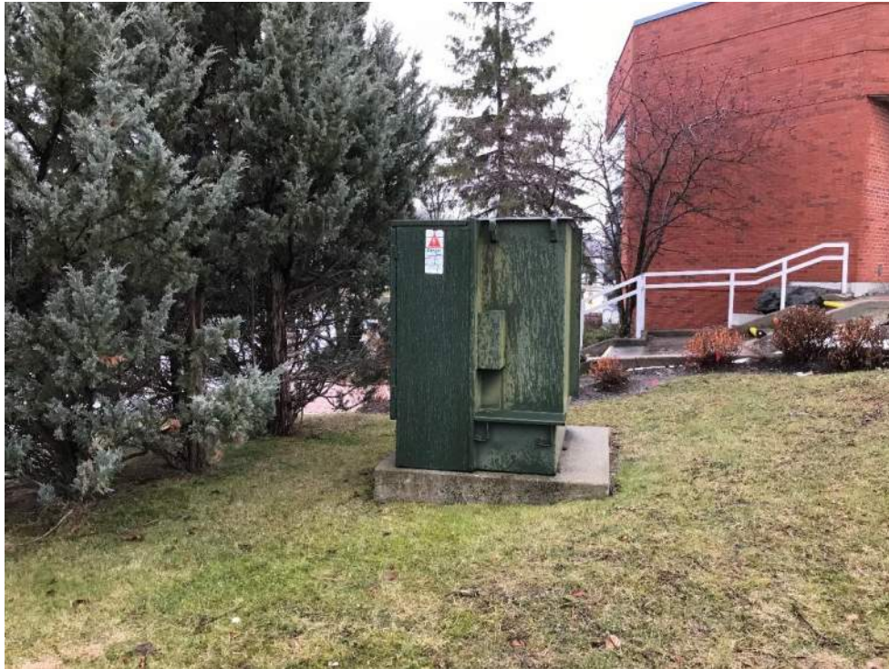
Photo 3 – Photo showing the pad mounted transformer east of the building
