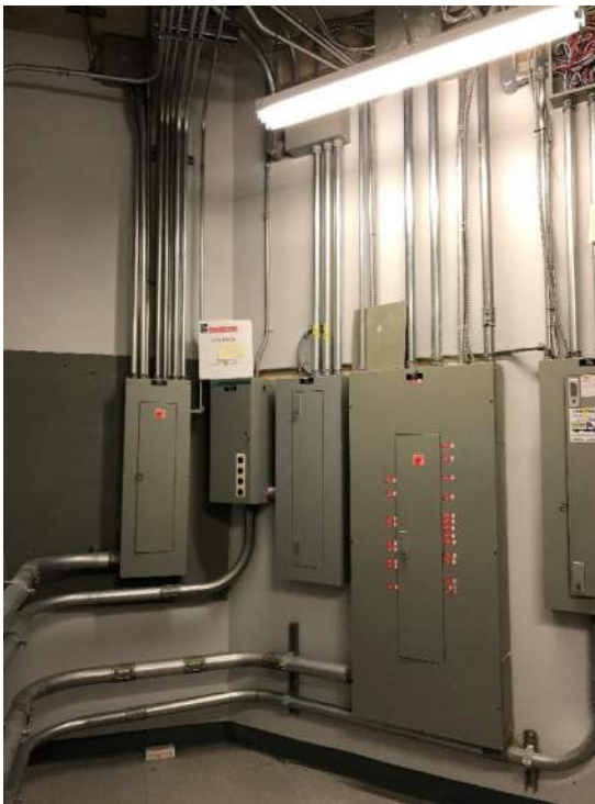
Photo 14 - View of the electrical room on the lower level of the building
