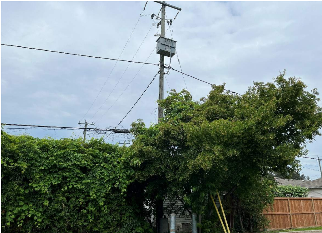
Photograph 4: Pole-mounted transformer along western property limits.
