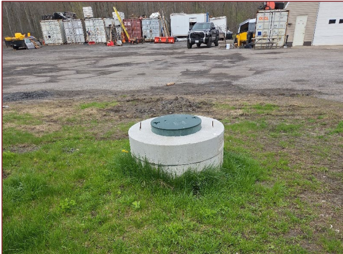
Photograph K11 – Looking west at water well. Sea cans and small shop are seen behind.
