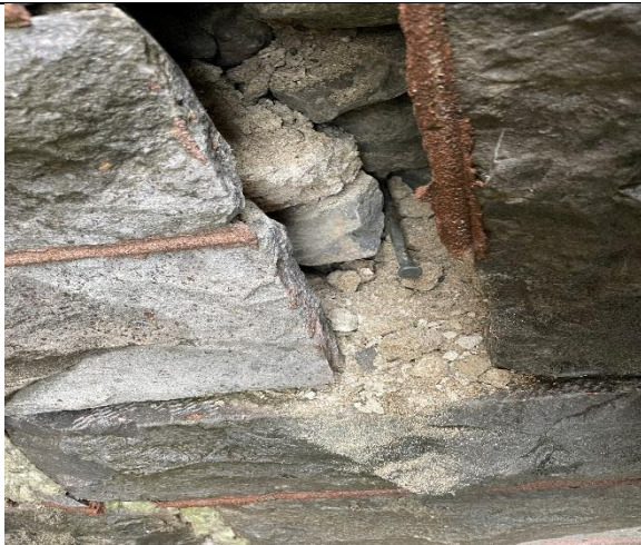
Photo 8: Large fracture on east wall of north annex at chapel. Large voids, loose stone gallets and sand in wall core.
