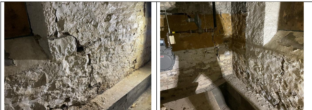
Photo 1: Crack in east chapel wall – basement level concrete benching.
