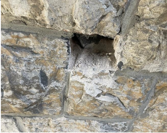
Photo 5: West wall of House. Core behind small stone has soft lime mortar bonded to adjacent stones.
