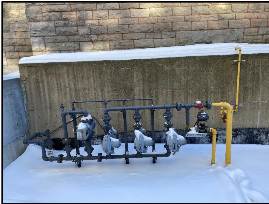
Photo 9: Natural gas infrastructure on the north side of the subject building
