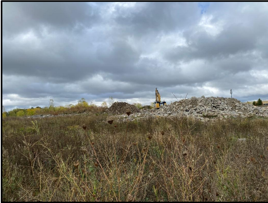
Photo 9: Excavation and stockpiling of boulders occurring on the north side of the Phase I Property, picture taken facing west.
