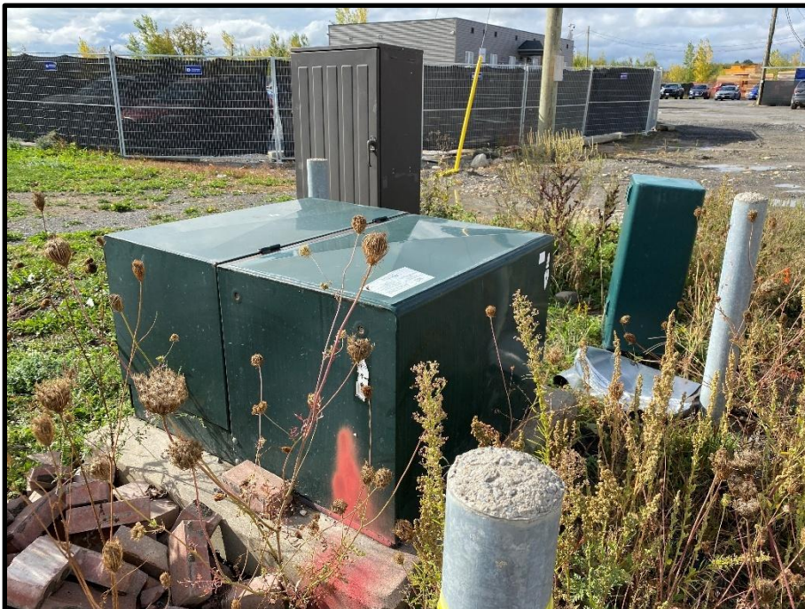
Photo 8: Pad-mounted transformer at the northeast corner of the Phase I Property, picture taken facing southwest.
