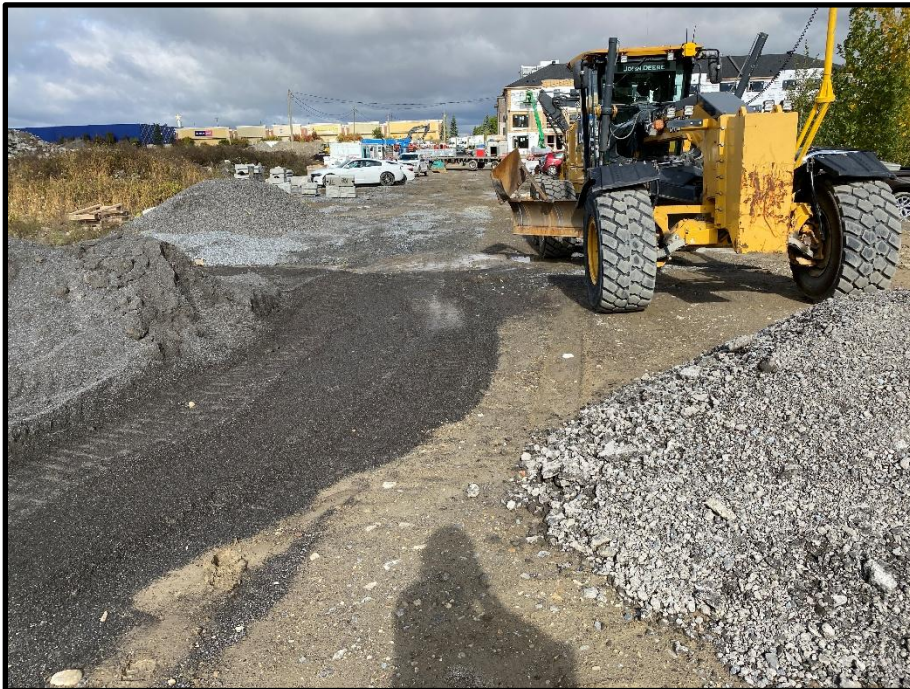
Photo 10: Engineered granular materials on the north side of the Phase I Property, picture taken facing north.
