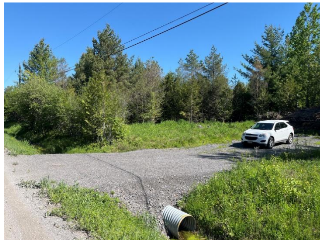
Photo 11: Entrance to Subject Property from David Manchester Road in MEGM3-8. Facing northeast.
