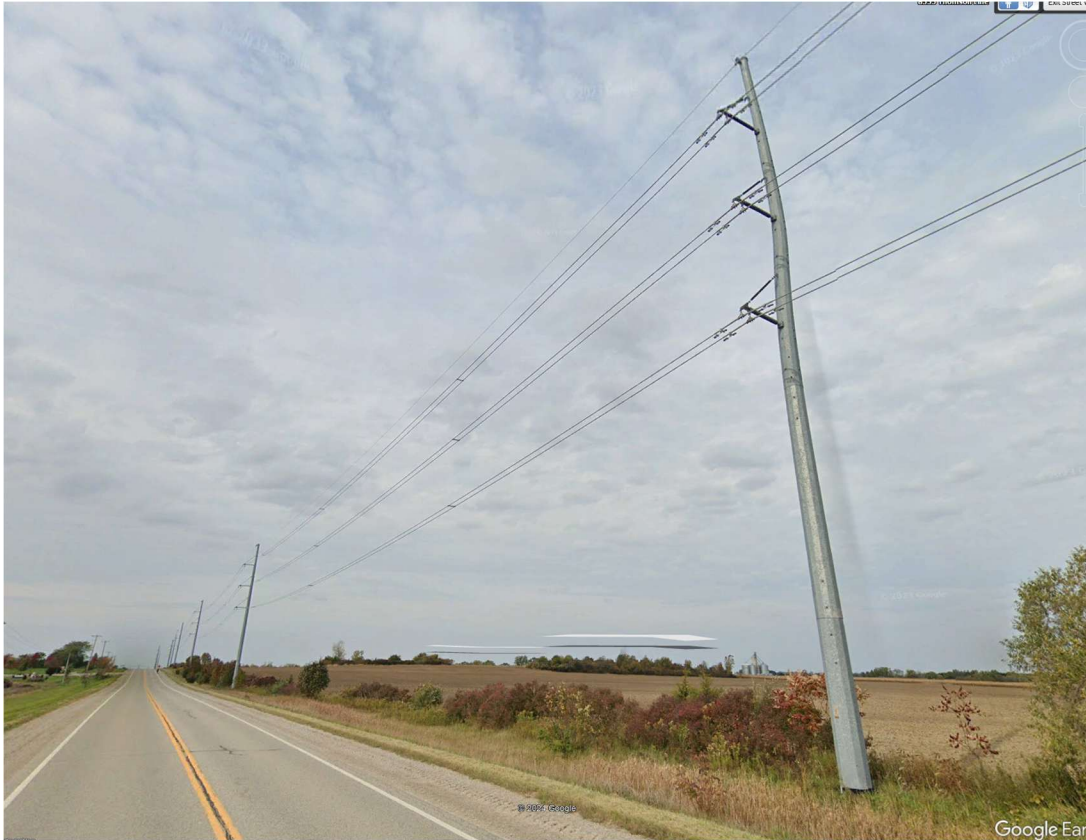
Figure 3.2.1 above is an example of a 230 kV monopole T-Line similar to the Trail Road design
