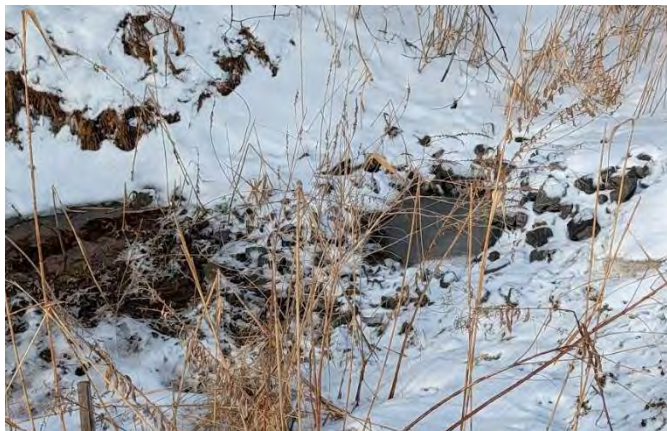
Photo 1: Image taken at culvert south of Navan Road on March 26, 2026. Weather around 2 degrees with snow melting. No water was observe flowing from the culvert as noted by frozen surface water at culvert exit. Only standing water was observed in the drainage
