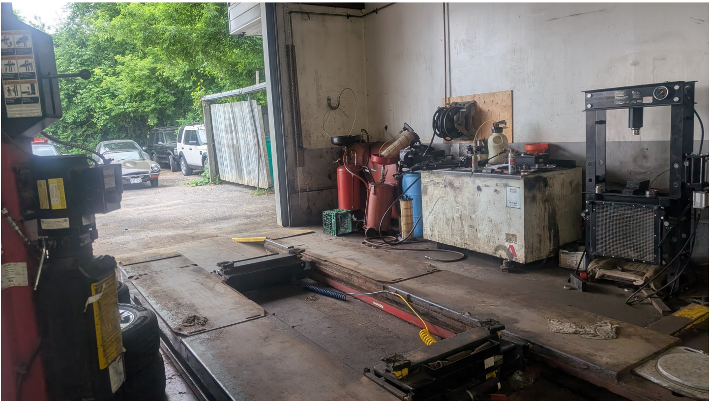
Photo 20 - Looking south towards the west building line of 1064 St. Laurent Boulevard. Waste oil AST and work bench tank can be seen along the building line.
