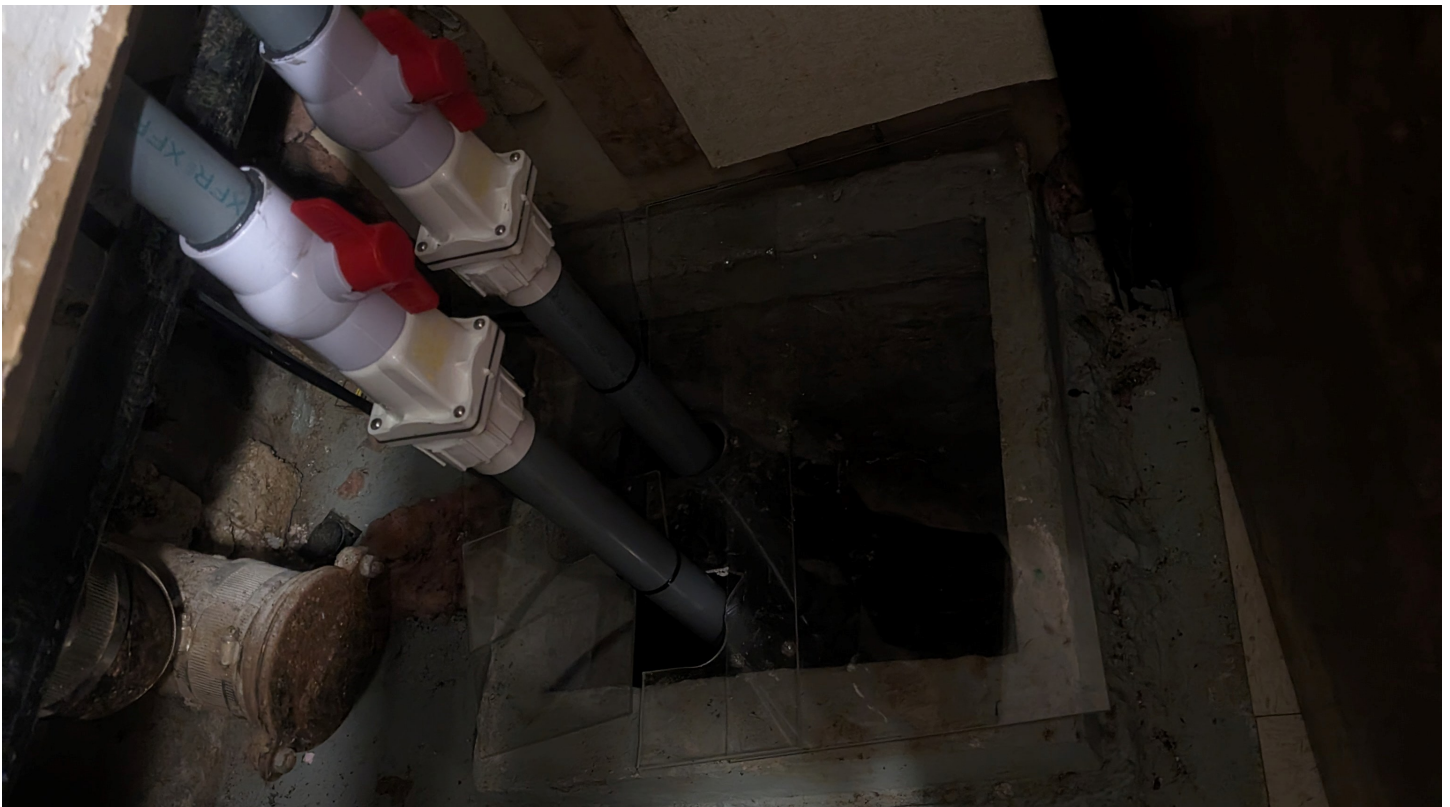
Photo 4 - Looking north towards a sump pit inside the basement of 1052 St. Laurent Boulevard.
