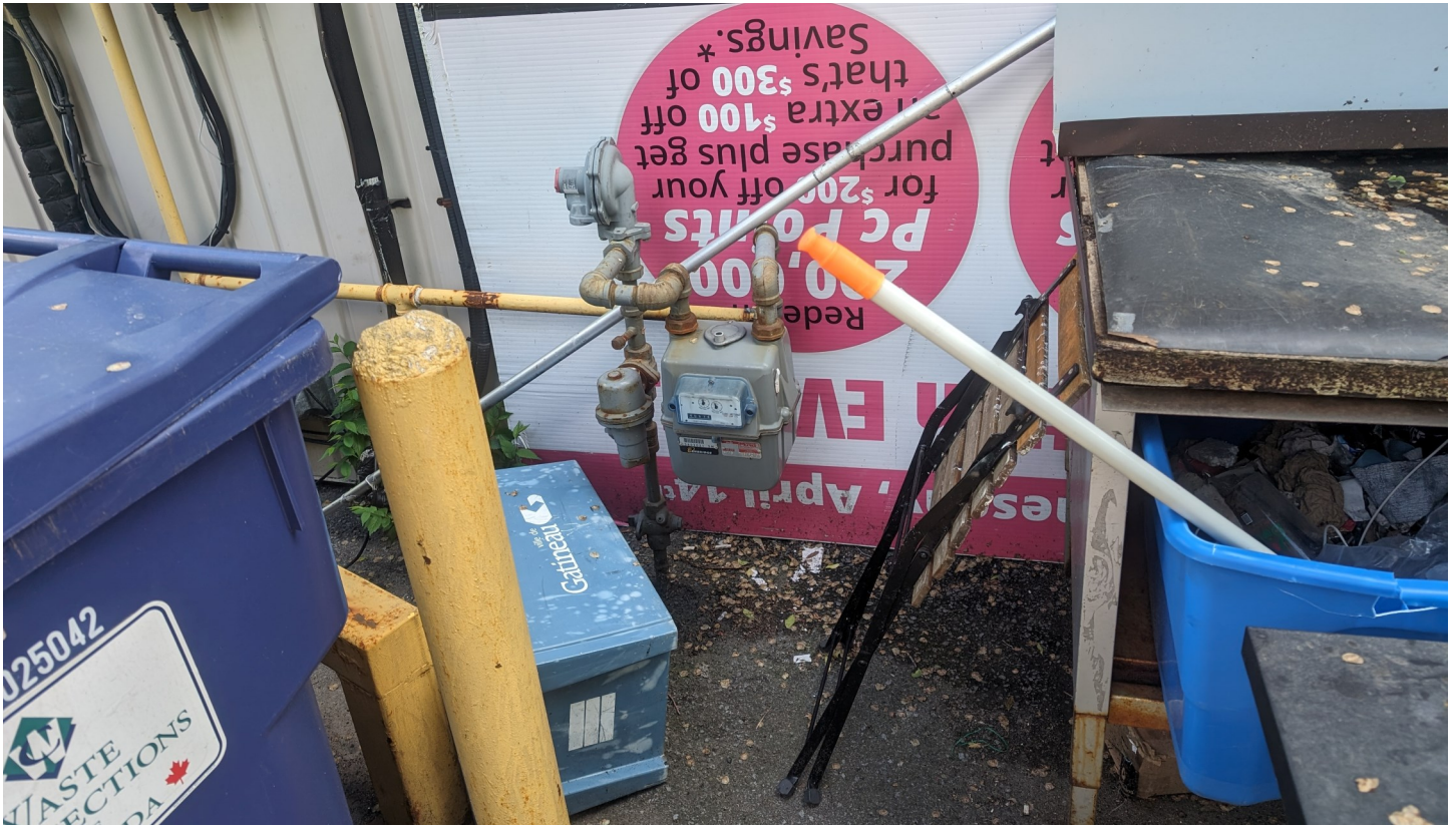
Photo 5 - Looking east towards the natural gas meter for 1052 St. Laurent Boulevard.
