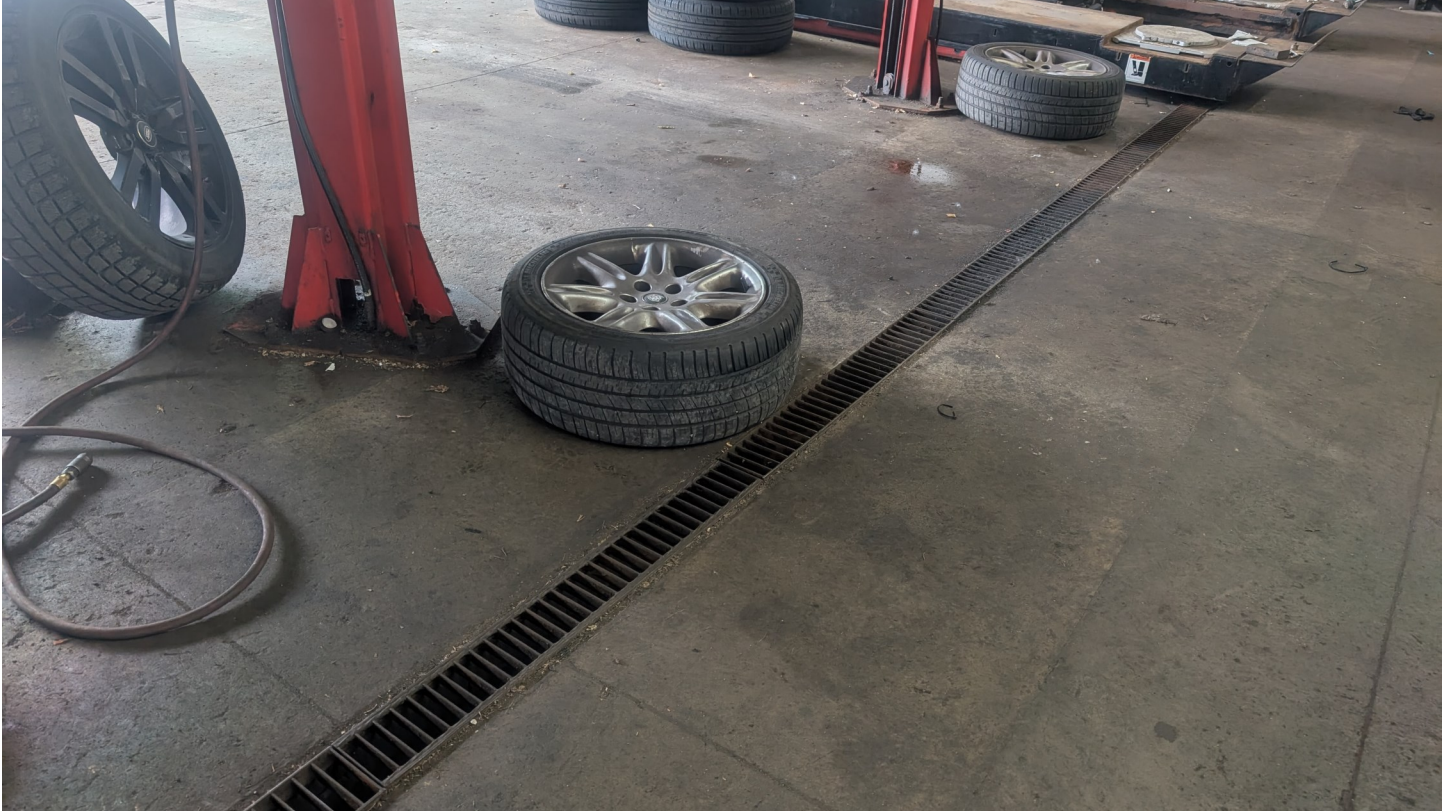
Photo 19 - Looking south/southeast towards the floor drains which discharge into the oil water separator at 1064 St. Laurent Boulevard.
