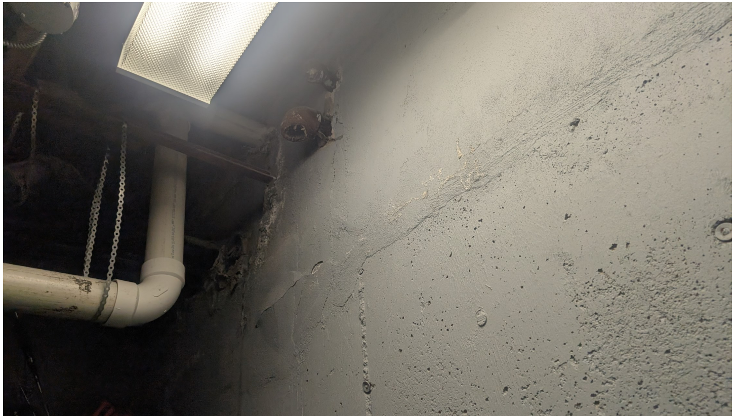
Photo 6 - Looking west towards the west building line where two pipes (likely vent pipe and fill pipe) were located.
