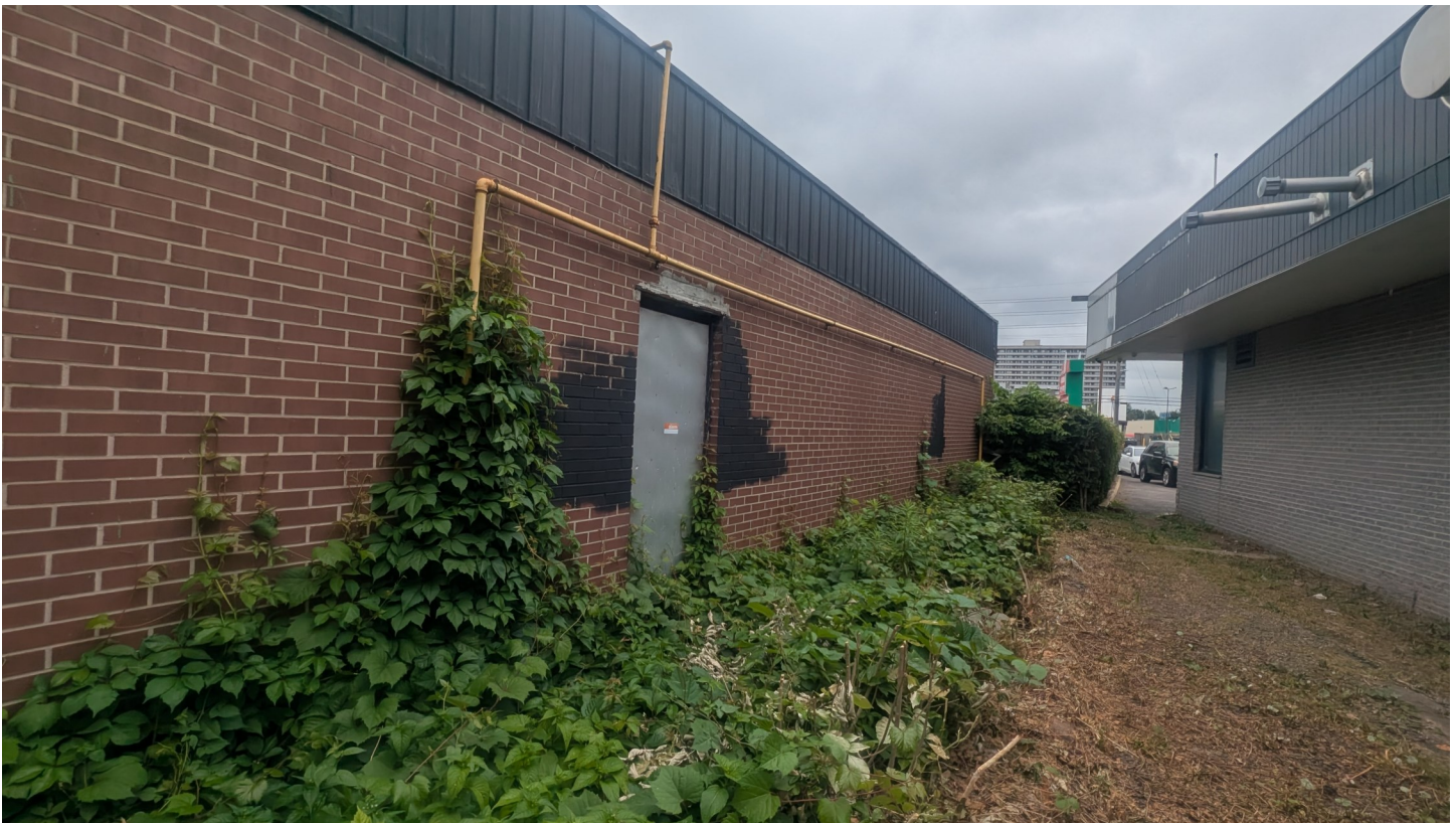
Photo 12 - Looking east from between 1060 St. Laurent Boulevard and 1064 St. Laurent Boulevard. Natural gas meter for 1060 St. Laurent Boulevard is to the left.
