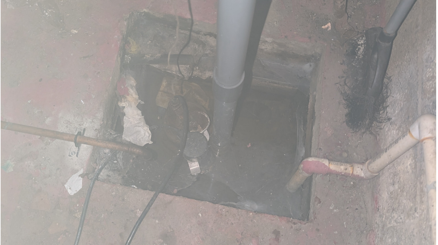
Photo 11 - Looking west/southwest at the sump pit located in the basement of 1060 St. Laurent Boulevard.
