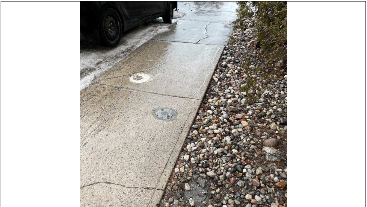
Photo 016 View of multiple groundwater monitoring wells along the eastern sidewalk of the Phase One Property (along Parkdale Avenue) (facing south).
