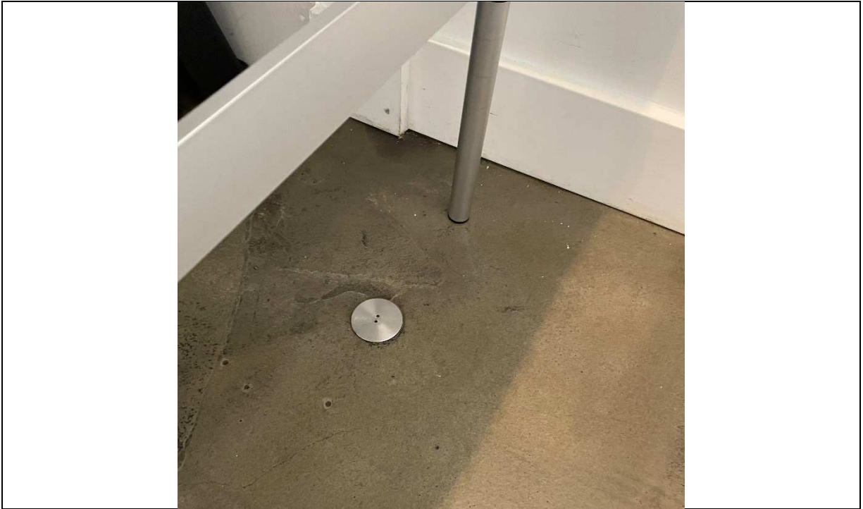
Photo 005 View of suspected soil vapour probe under tattooing table in Railbender Tattoo and Shades & Art Gallery located at 3 Hamilton Avenue North (the Phase One Property) (facing down).
