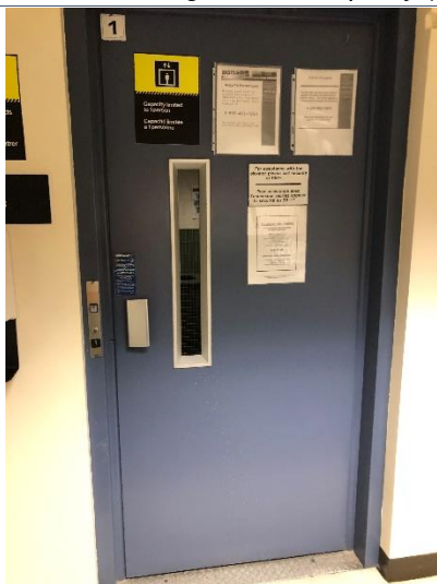
Picture 3 – Hydraulic Elevator Inside Office Building
