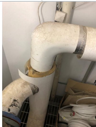
Picture 4 – Pipe Wrapping Within 2 nd Floor Mechanical Room of Office Building
