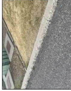
3 DEGRADED, CRACKS & UNEVEN SIDES
