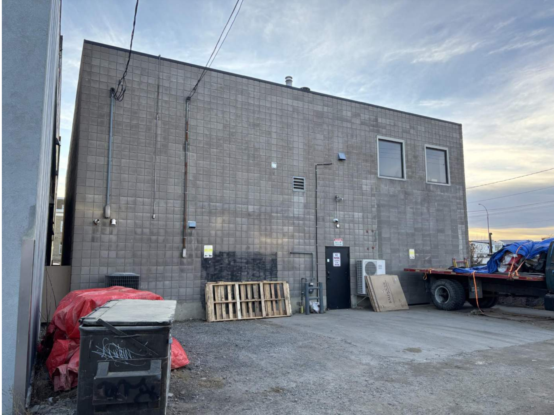
OVERHEAD UTILITY LINE CONNECTION TO BUILDING
