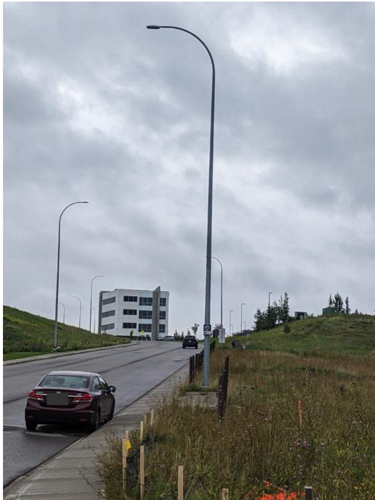
V7. DETAIL OF OVERHEAD POLE
