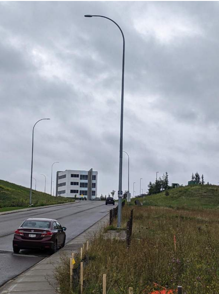
V7. DETAIL OF OVERHEAD POLE
